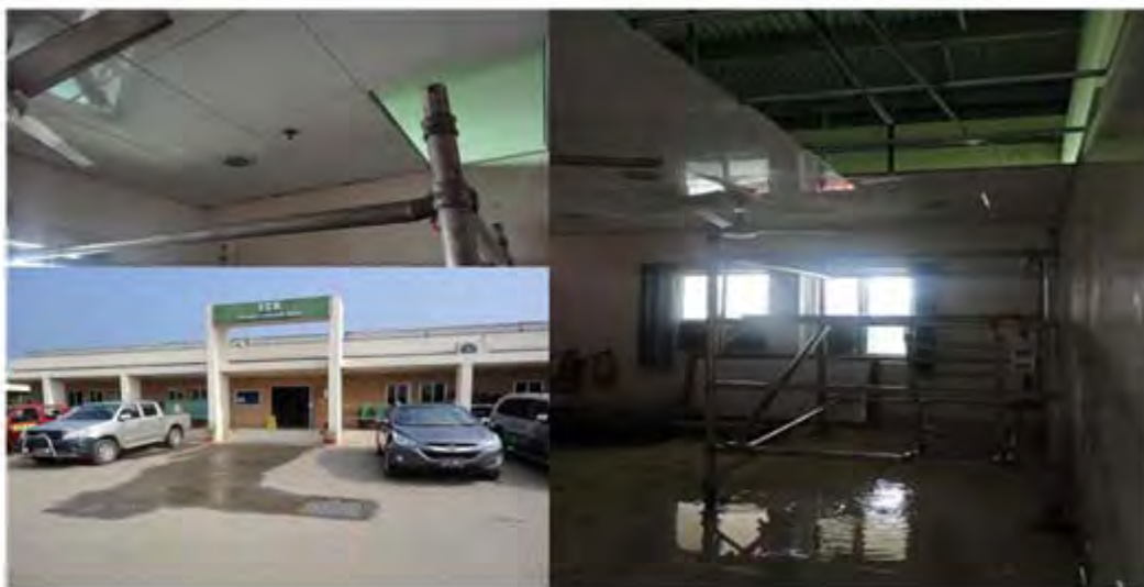
Figure 5.1 Picture of the Incident
