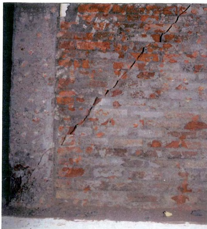
Fig.: 3.32 The close up view of crack through the masonry infill.
