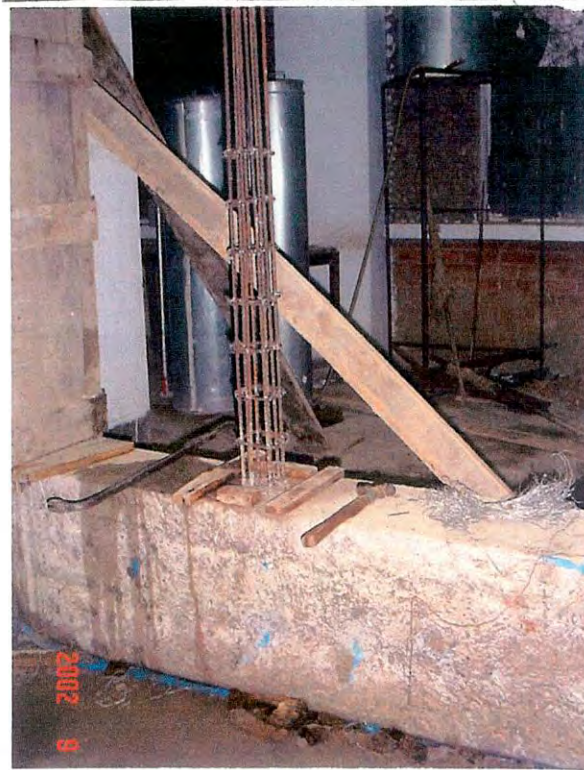
Fig: 3.9 Close up view of the reinforcement in column of the infilled frame.
