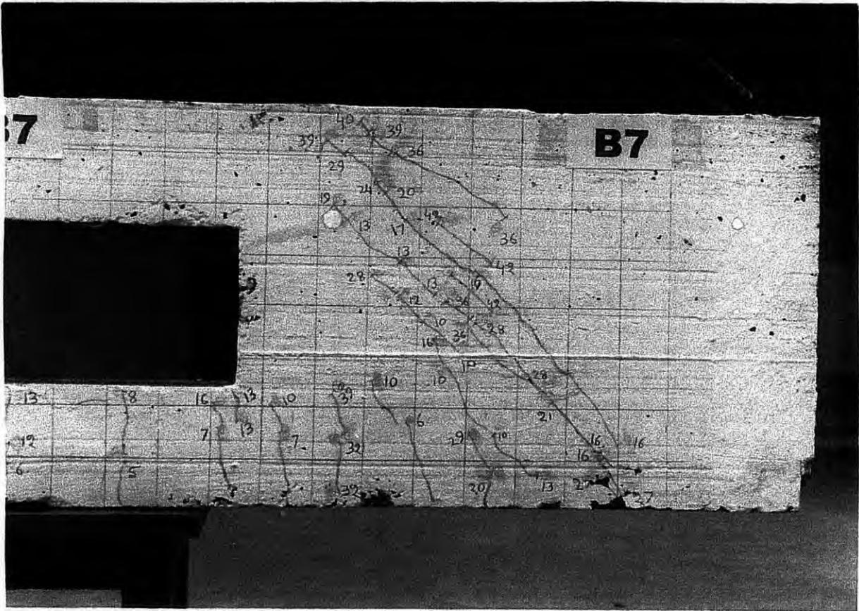
Figure 5.4g Crack pattern of beam B7
