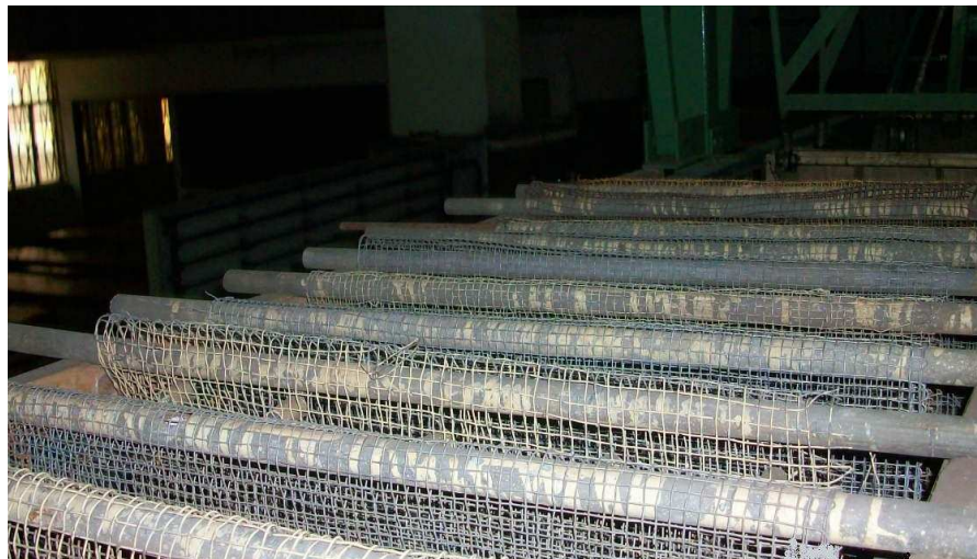
Photograph 4.2.3: Weir Mesh (Screen)
