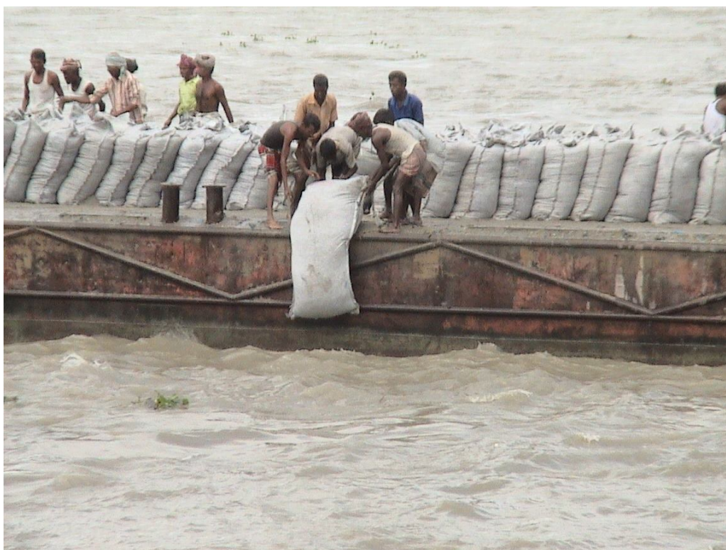
Photograph 2.1: Geobags are being dumped for toe protection at Sirajgonj Hard Point (Field visit on 21.07.2011)
