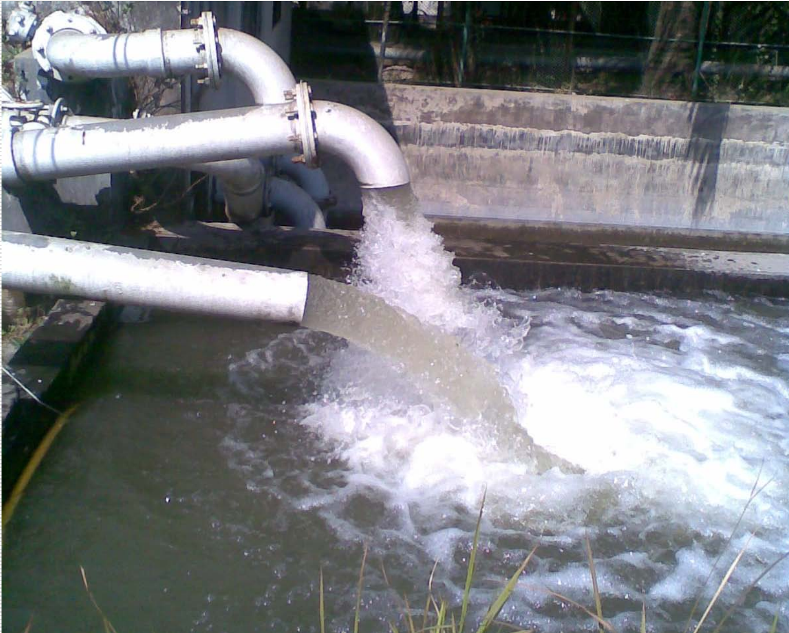
Figure : Water recycling pump.
