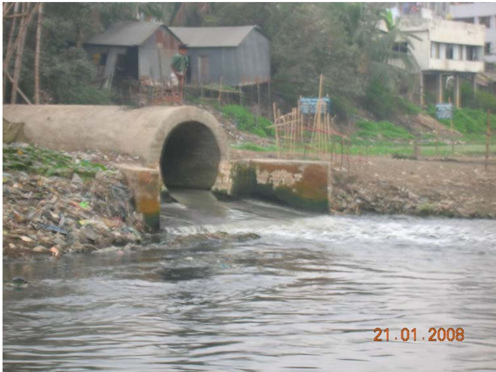
Photograph 3.6: Storm sewer coming from Mouchak-Rampura area and discharging into Hatirjheel near Rampura bridge (Q7)
