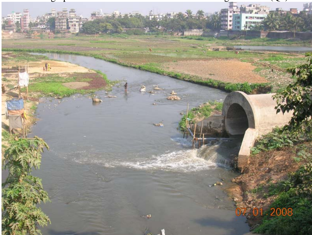
Photograph 3.2: 96-inch diameter storm sewer outfall located immediately to the east of Tongi Diversion Road (Q2)
