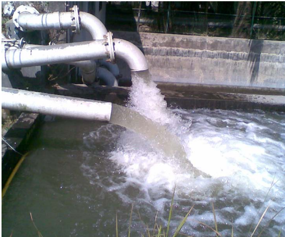
Photograph 4.19: Water recycling pump.
