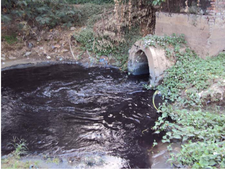
Photograph 3.3: Out fall located at the North-west Tajgaon diversion road (Q4).
