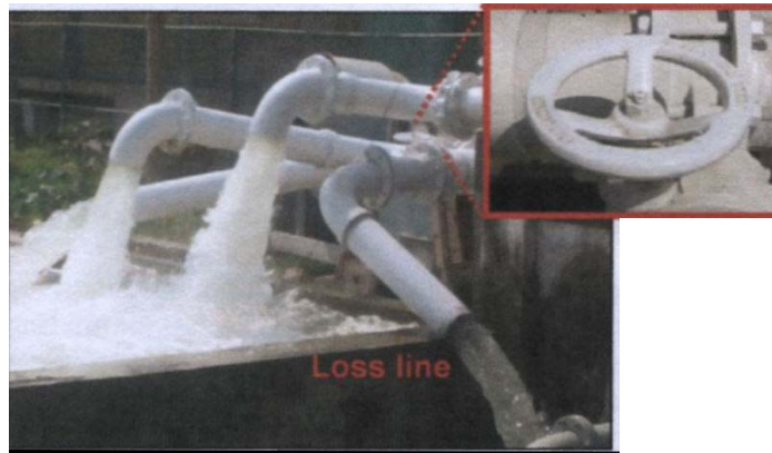
Photograph 4.11 : The loss line (l) with valve (in frame) and flow depth control by means of the tail gates(r)
