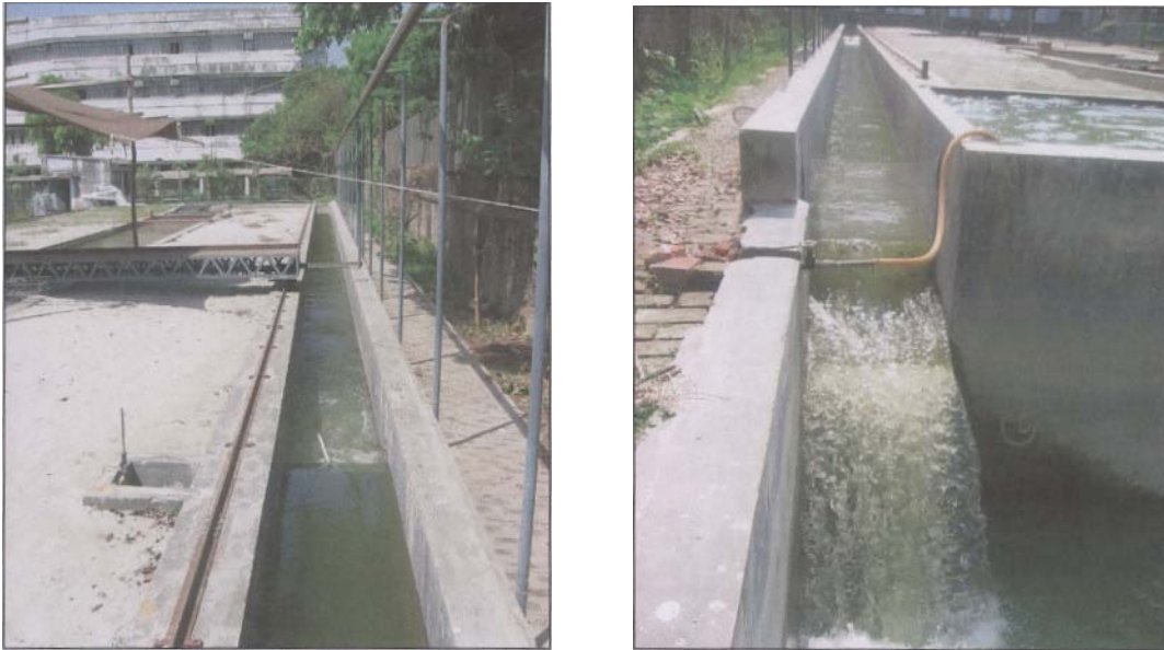
Photograph 4.9: The re-circulating canal (with weir) seen in downstream (I) and upstream (r) direction
