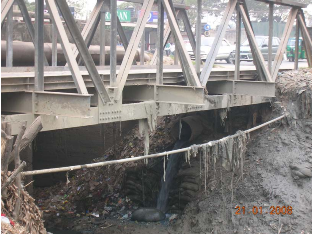
Photograph 3.8: A pipe discharging industrial wastewater underneath the bridge on Gulshan-Tejgaon Link Road
