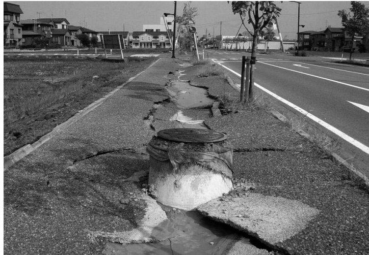
Figure 2.10: Liquefaction in a Sewer Line (Chuetsu Earthquake)
