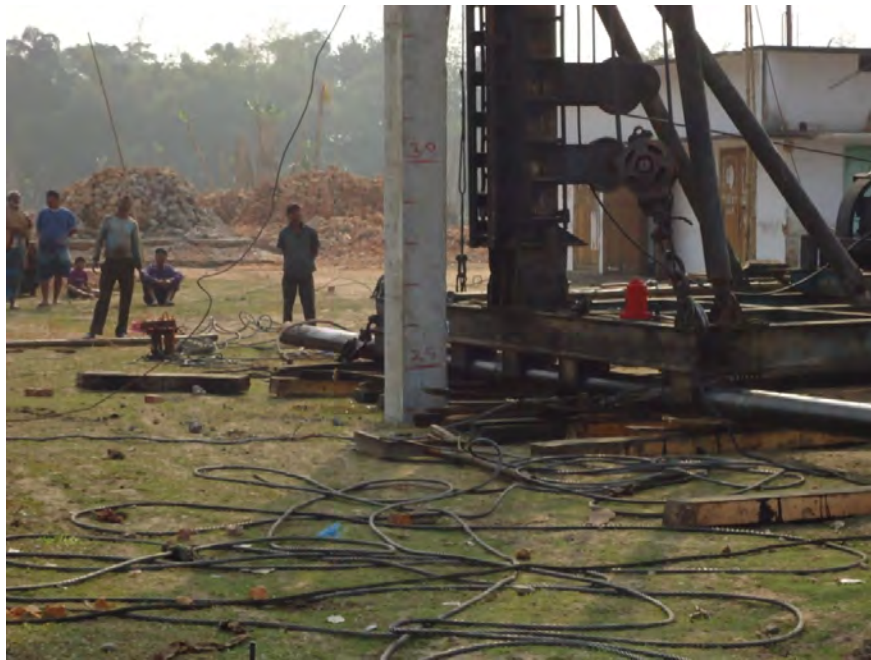
Figure A2 Spliced Precast RC Concrete Piles before casting and during driving (Source: PWD)
