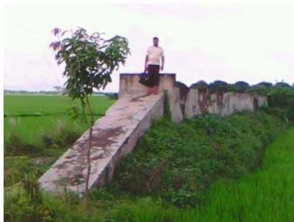
Siphon and RCC Canal on Ground of Nayagola-Mohananda Irrigation Subproject
