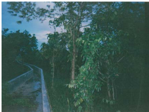
RCC Canal start from Sump of 2nd lifting arrangement of Mohammadkhani Subproject
