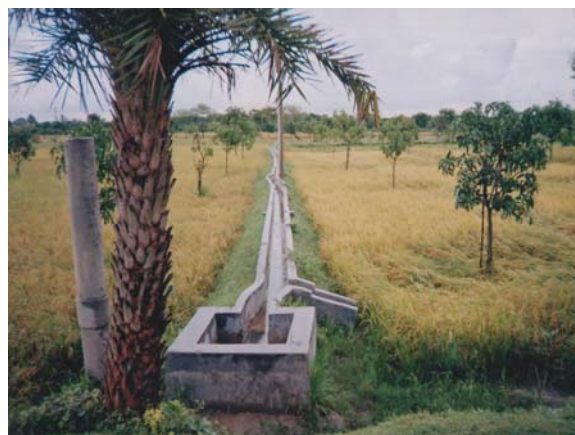
Outlet and field canal of Buried Pipe Irrigation system of Dariapur Subproject
