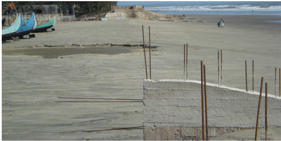
Figure C2: Washed out portion of Marine drive at Kalatoli, Cox's bazar
