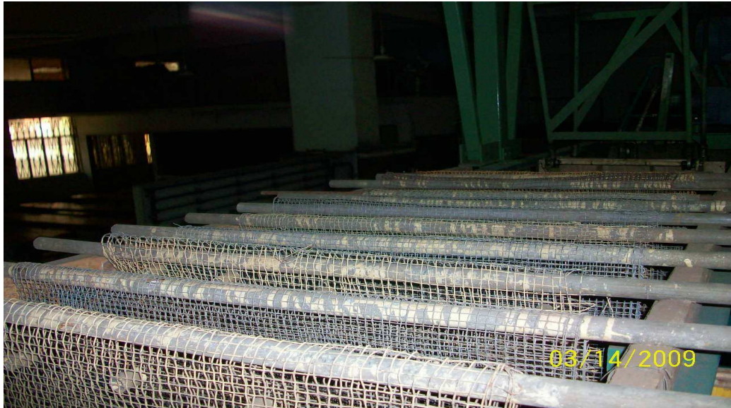
Photograph 3.4.6: Wire screens in the flume
