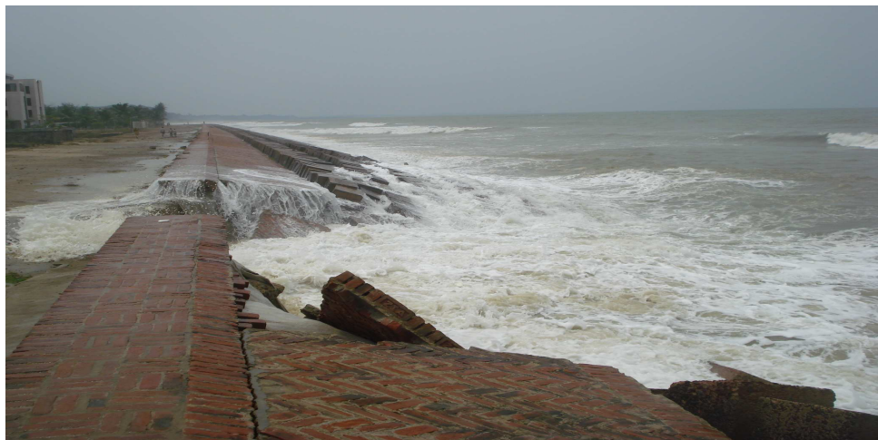
Figure C8: Wave attack at the Damaged portion of the embankment
