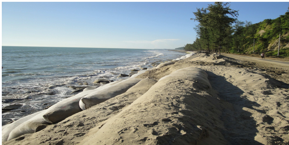
Figure C11: Destroying part of the Marine drive at Himchari, Cox's bazar
