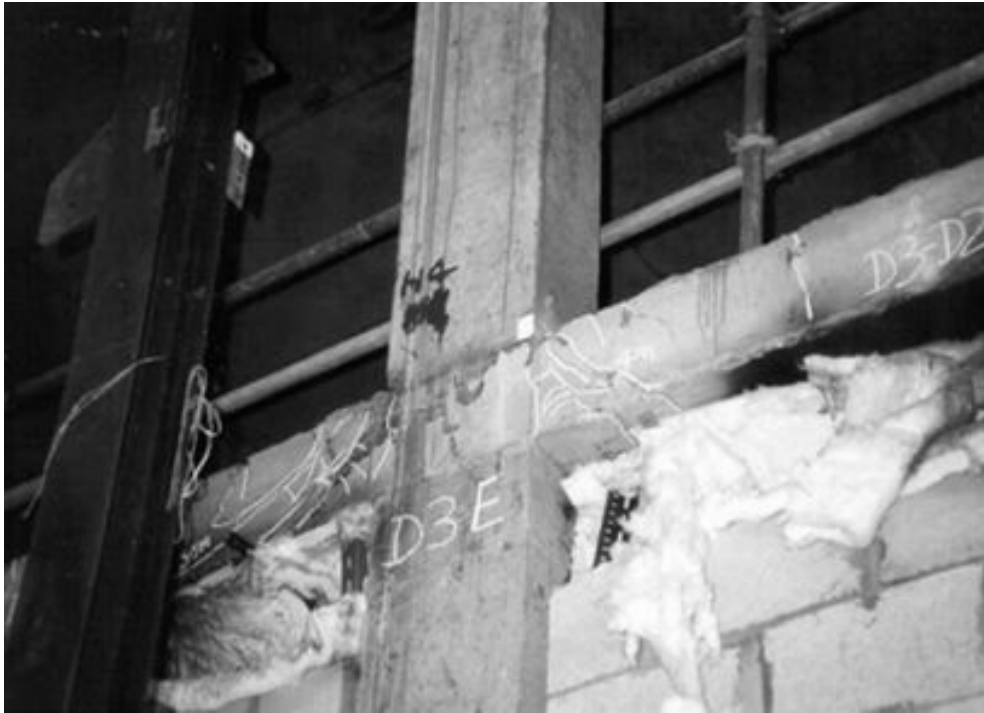
Figure 2.7 Cracking in the proximity of column
