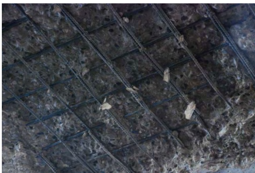
Figure 2.5 View of a spall on a fire-damaged concrete slab soffit.
