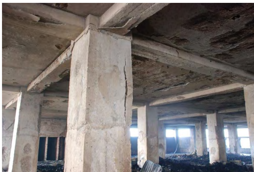
Figure 2.6 Interior column spalling
