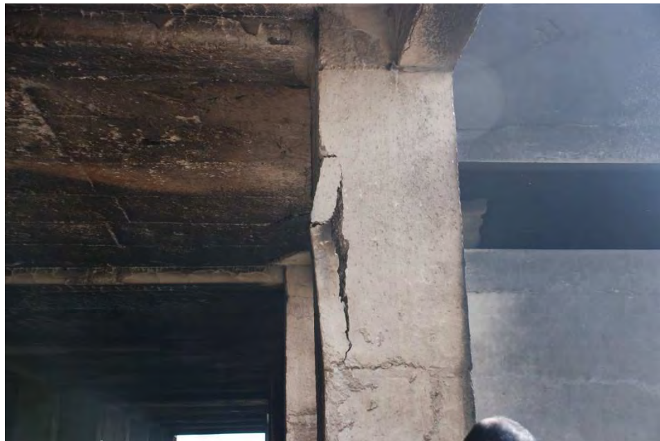
Figure 2.8 Longitudinal cracking in column
