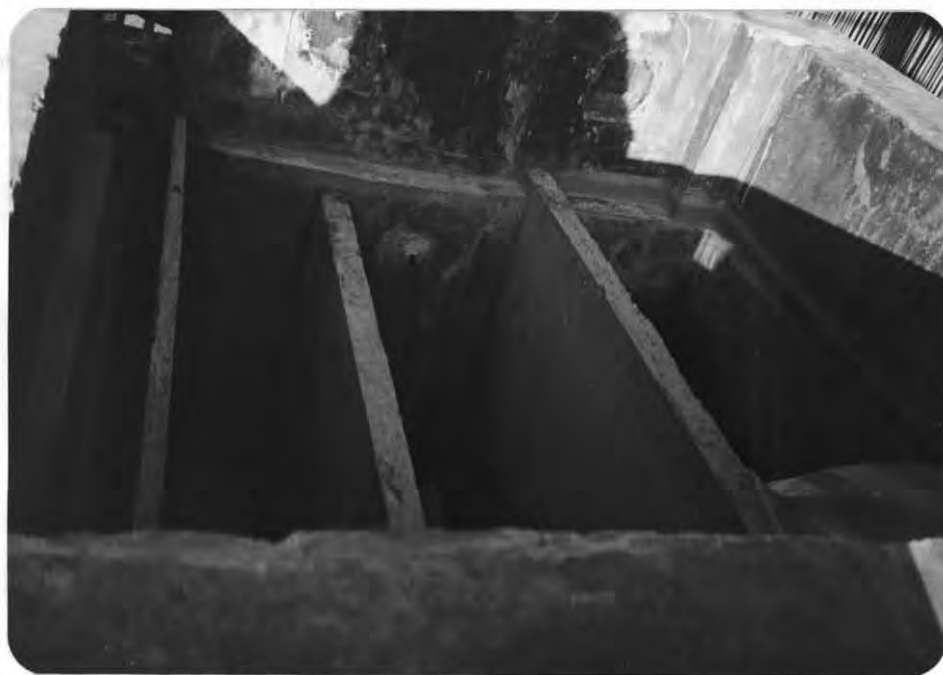
Plate No. 3 Modified Iron Removal Plant showing Different Chambers
