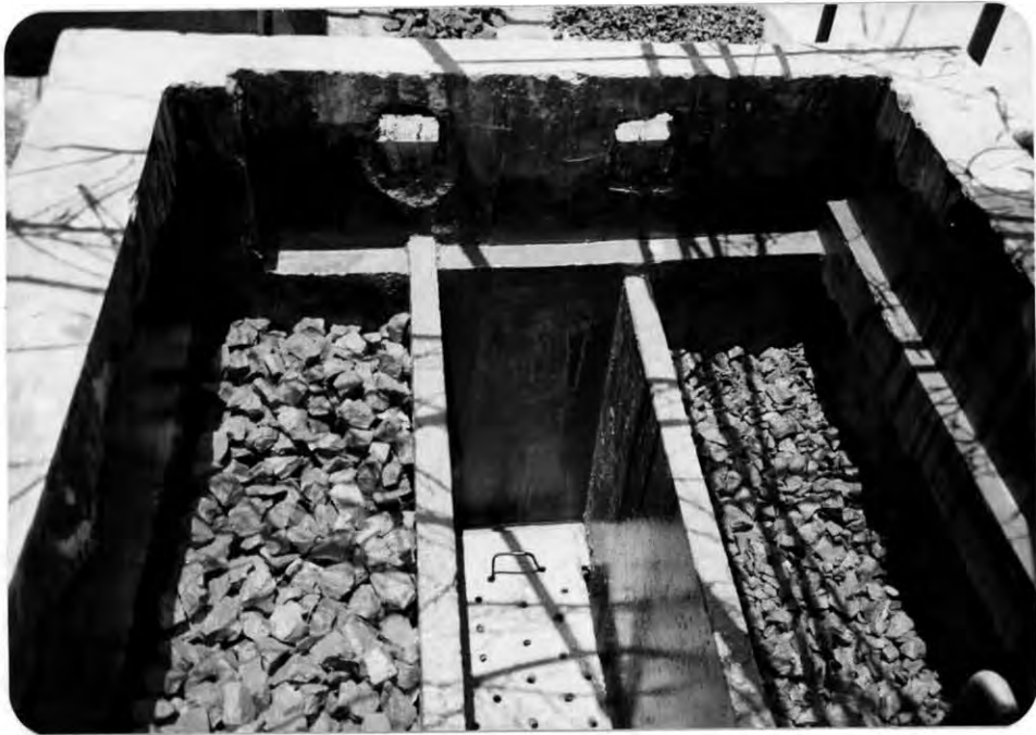
Plate No. 1 Iron Removal Plant showing Different Chambers with Media
