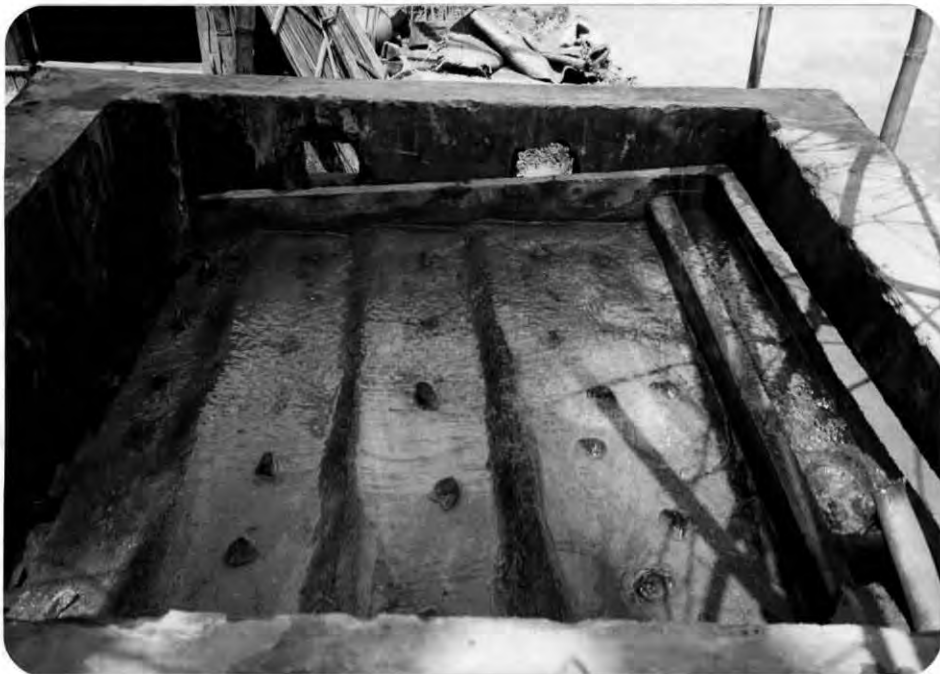
Plate No. 2 Iron Removal Plant showing the Aeration Chamber
