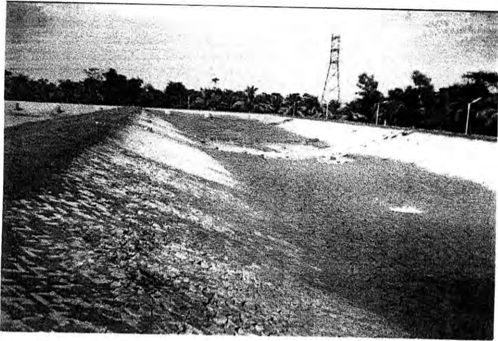
Sedimentation basin of the plant (Basin was used for desludging)
