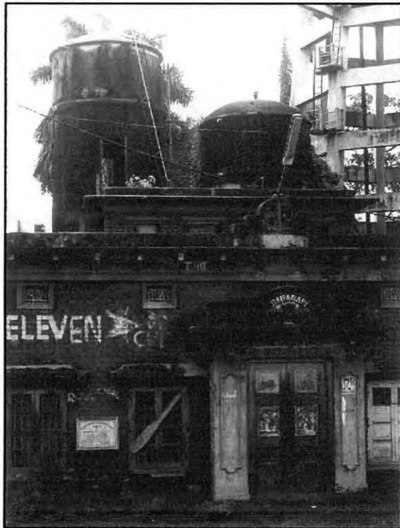
Photograph-03 Iron & hardness removal plant, installed in 1937, the first effort to safe water supply
