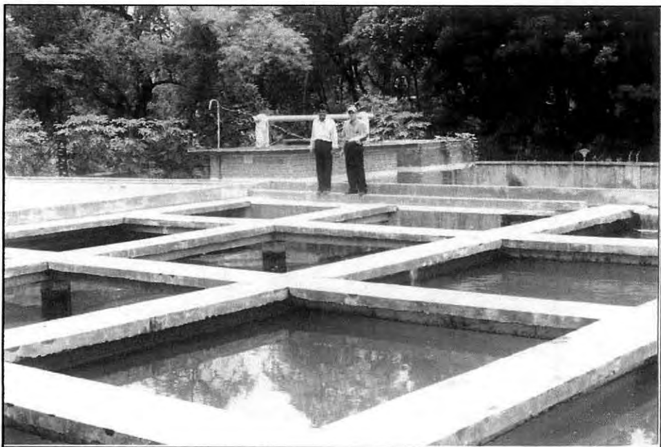
Photograph-04 Sedimentation tank of Water Treatment Plant near BDR camp
