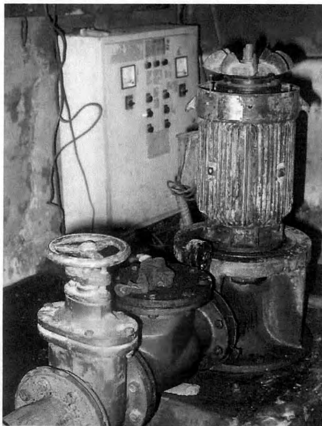
Photograph-09 Pump House (Turbine) at PN Girls School.
