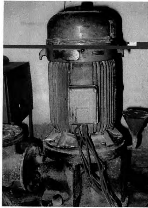
Photograph-10 Pump House(Submersible) at Hatem Khan(Hemnati Kumari Water Works Compound)
