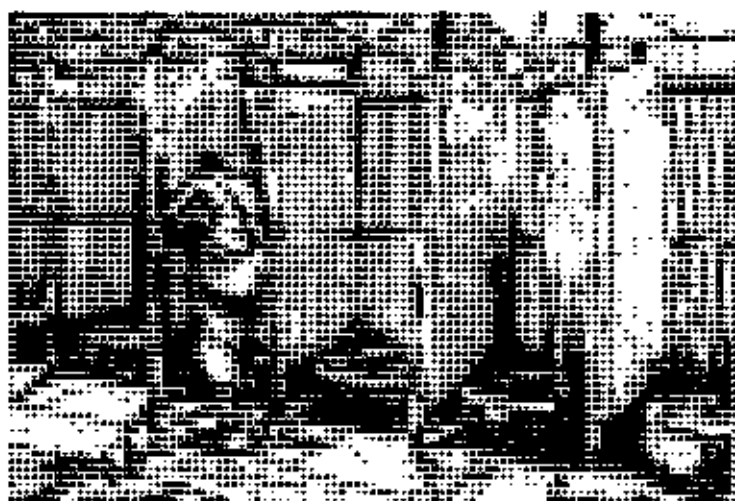
Plate: 14 Unsatisfactory structural and visual conditions of community latrines provided by Plan International in Agargaon usually fill up by excreta. Acceptance for women is a question to use these latrines.
