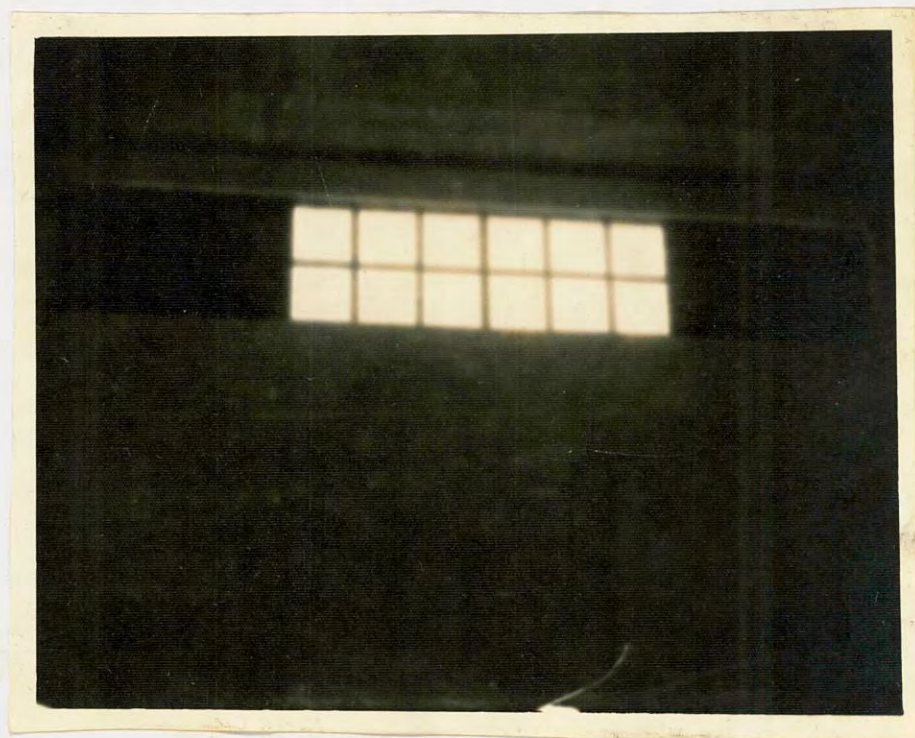
Fig. 4.4 Ventilation system at Daudkandi which permit entry of rain water into the godown.
