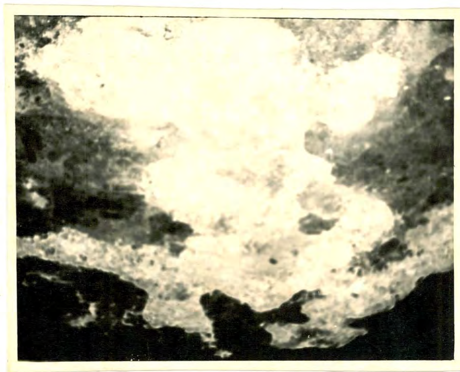
Fig. 4.2 Effect of urea on floor slab.
