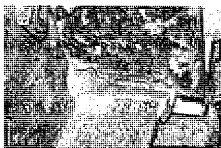
a. Fracture at Weld Zone
