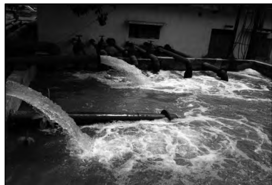
Figure A.34: Pump for Delivering Water to the Sump
