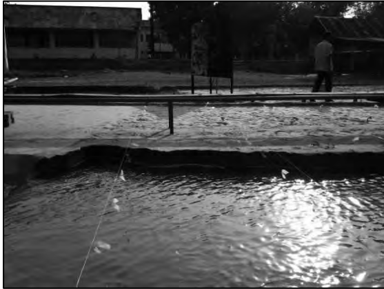
Figure A.41: Bank Erosion at D/S
