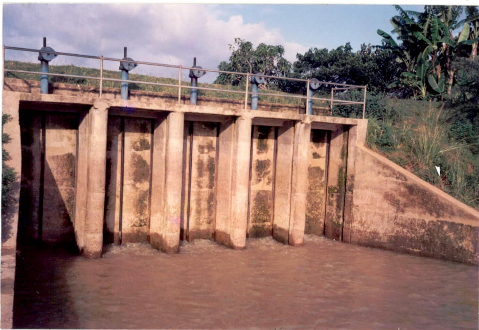
Photo 2: River side view of Chuller Khal regulator which is in good operating condition (Date : 16-8-94)
