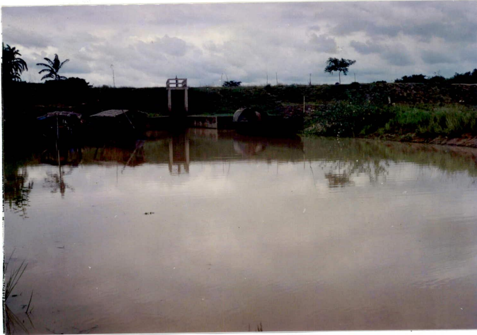
Photo 3: River side view of 1 vent Suktajuri Khal Regulator. The structure prevents boat traffic (Date : 16-8-94)
