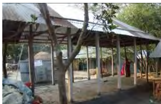
Figure 5.3: Rebuilding of a traditional house with precast RCC post and CI sheet roof. *
