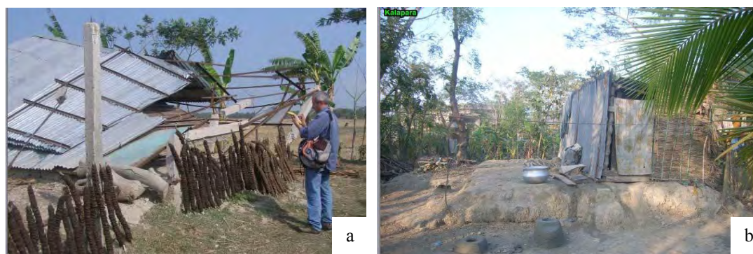
Fig 5.4. a. Damage of built-up structure, Kalapara . (The photograph was taken on 20 Jan, 2007 ; 1 months after cyclone Sidr , (source: GoB-MoFDM, 2008, p 155)
