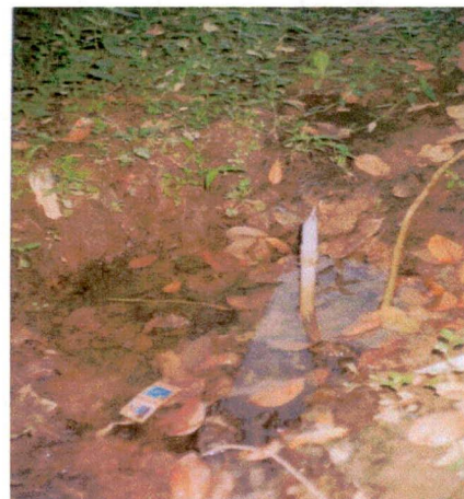
Figure 5.13: Air releasing pipe (South Chayabithi, Date: 23-11-02)
