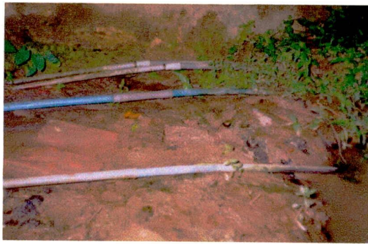
Leakage of pipelines (South Chayabithi, Date: 22-11-02)
