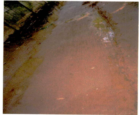
Leakage water overflow a road (South Chayabithi, Date: 22-11-02)
