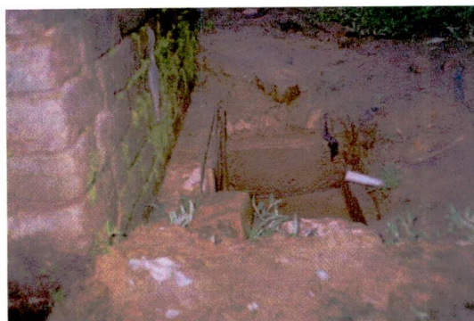
Yard connection without water (Boruda, Date: 23-11-02)
