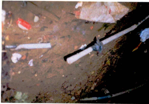
Breakage of pipelines (South Chayabithi, Date: 22-11-02)
