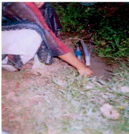
Figure 5.12: Releasing airlock (South Chayabithi, Date: 23-11-02)
