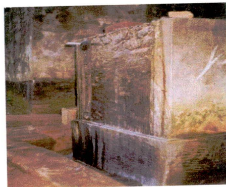
Overflow of storage tank (Jorpukurpar, Date: 22-11-02)
