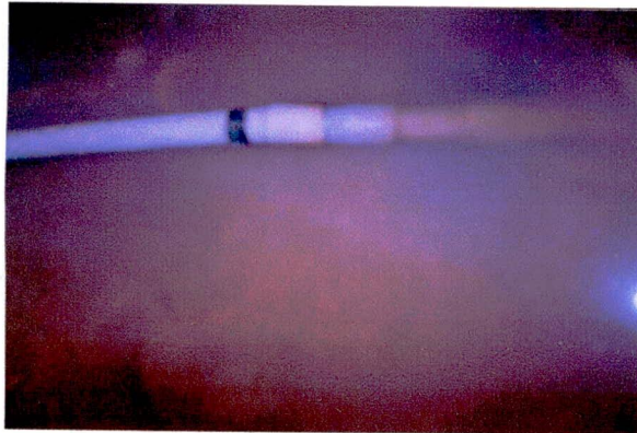
Leakage of pipeline (South Chayabithi, Date: 22-11-02)
