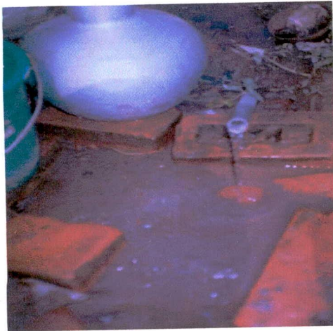
Low pressure at house connection (North Chayabithi, Date: 23-11-02)
