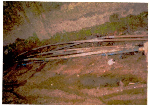
Leakage of pipelines (South Chayabithi, Date: 22-11-02)
