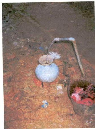
Low pressure at street hydrant (South Chayabithi, Date: 23-11-02)
