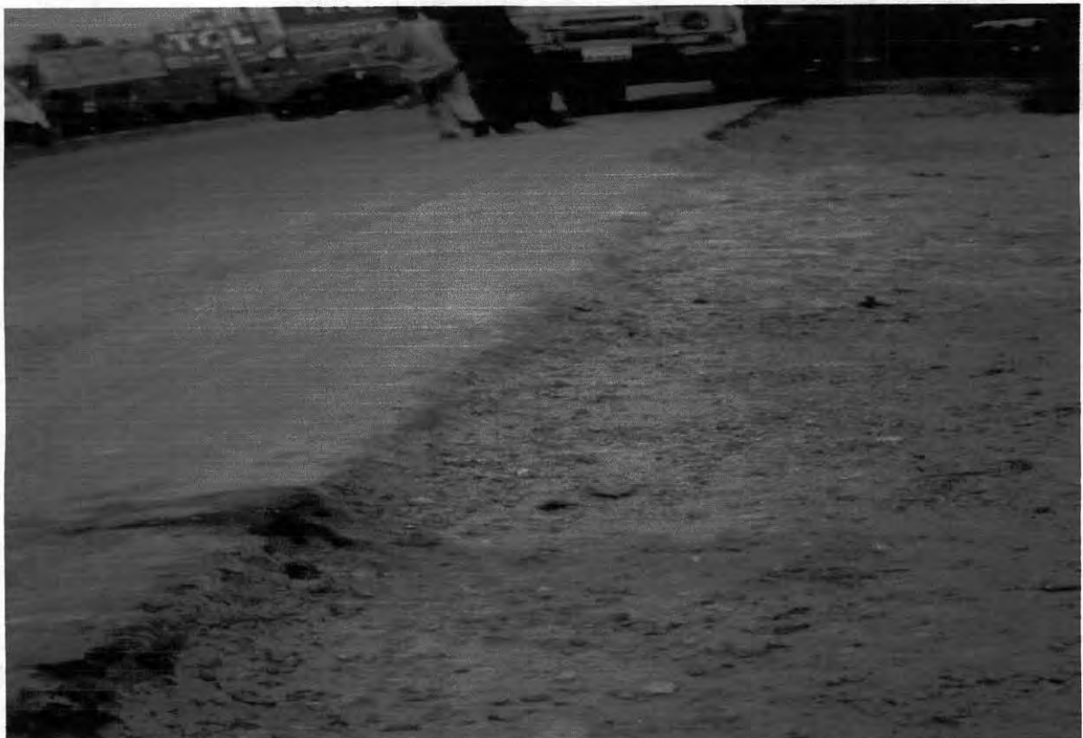
Figure B 4.6 Excessive shoulder drop along the Highway (3-5cm) is Very Hazardous Especially when Loaded Vehicle Reaches the Edge
