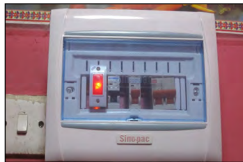
Picture 8.24: The circuit breaker used in the system.
