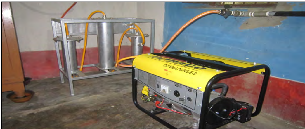
Picture 8.20: The gas generator with the biogas purifier.
