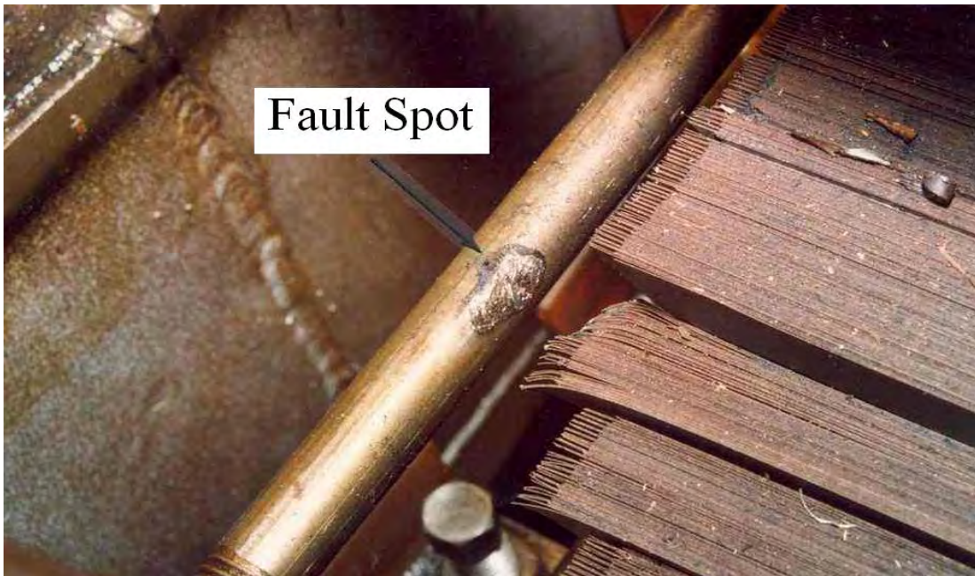
Figure 6.4: The position of the fault in the Core structure
