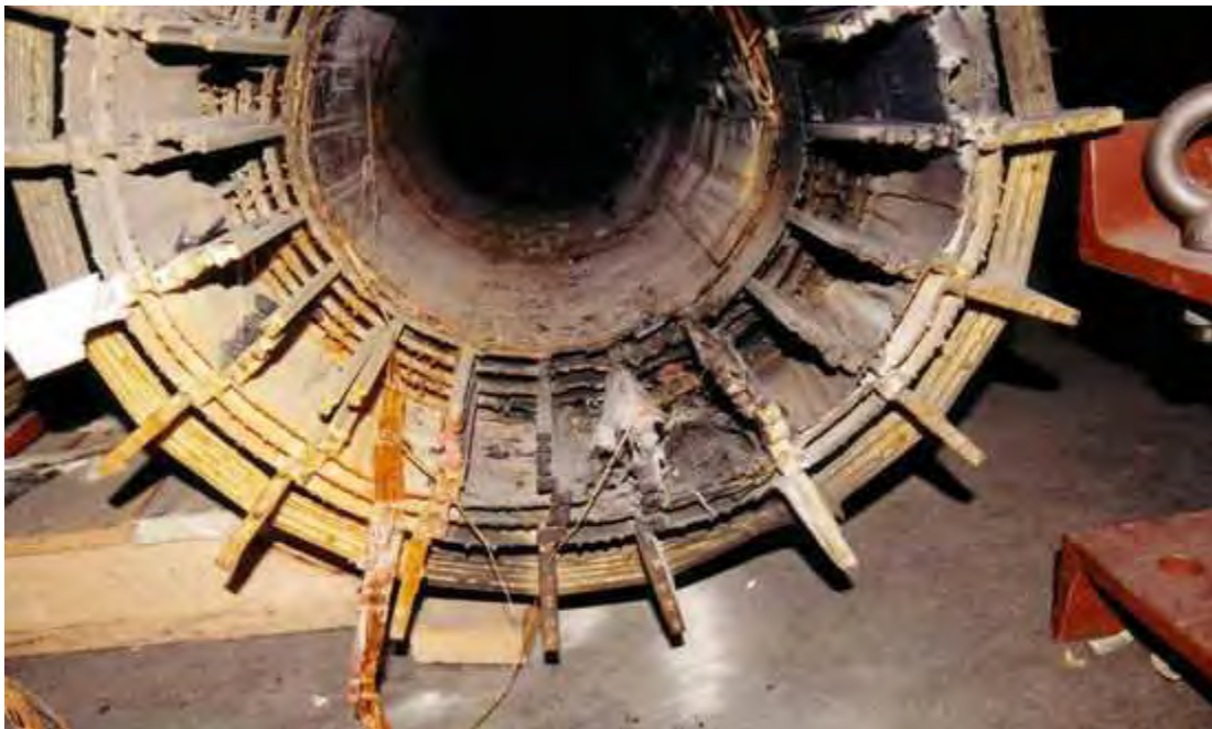
Figure 6.5: The damaged coil of HV A-phase (Red phase)
