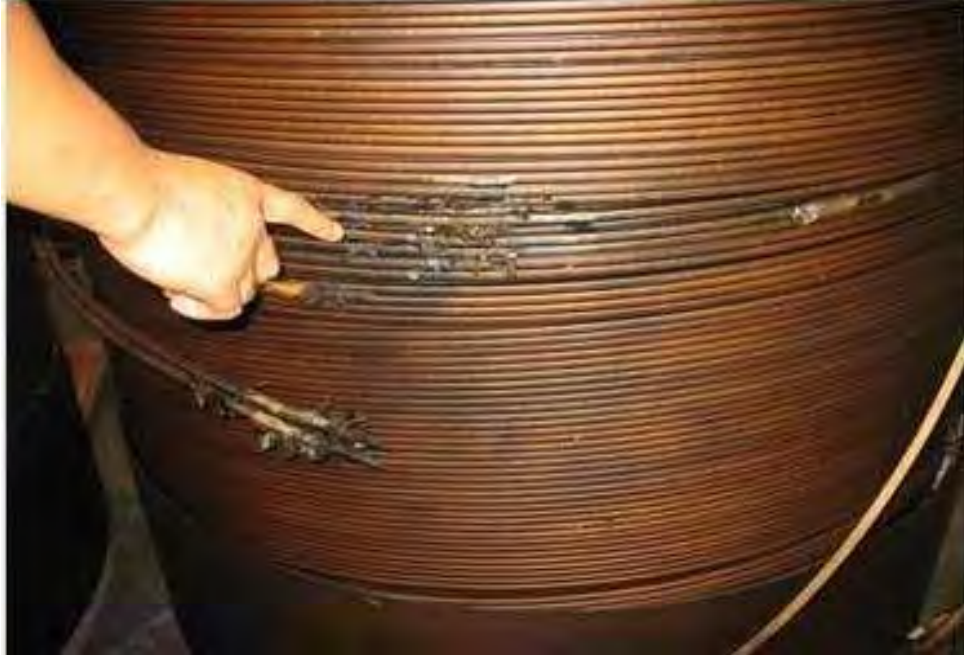
Figure 6.9: Damaged HV (phase-C) coil
