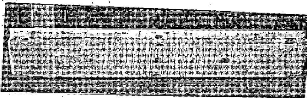
PLATE 5.5 CRACK PATTERN OF THE BOTTOM FLANGE AND SIDE WEBS OF THE ABOVE GIRDER
