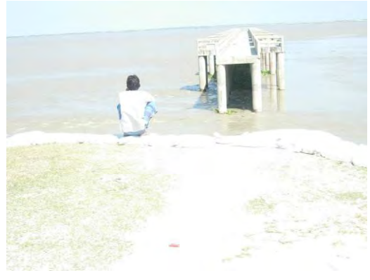
(b) Failure of bellmouth of the Baniajan spur (2007)
