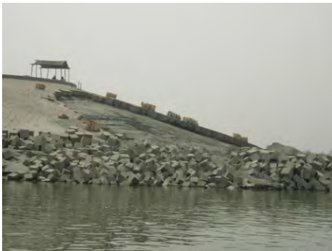
(e) Failure of the Sirajganj hardpoint (2008)
