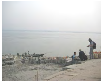
Figure 4.3: Failure part of the Sirajgang hardpoint (March, 2008)
