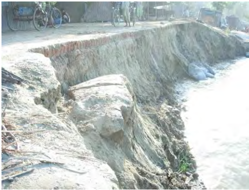
(c) Mass failure of the Ranigram groin (2007)
