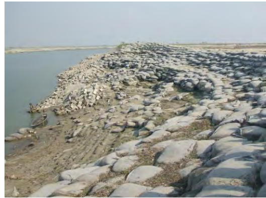
(d) Slip circle failure of the earthen shank of the Enayetpur spur (2007)
