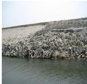
Figure 6.27: Failure of the earthen shank of the Enayetpur spur in July, 2008
