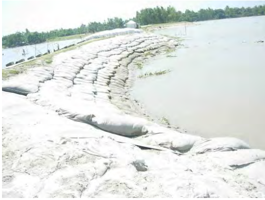
(a) Slip circle failure of the earthen shank of the Chandanbaisha spur (2007)
