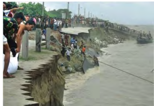
(f) Failure of the Sirajganj hardpoint (2009)
