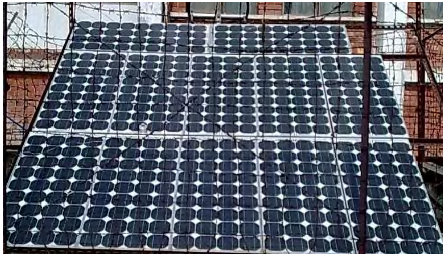
Figure 4.1 Solar Array consisting twelve solar panels
