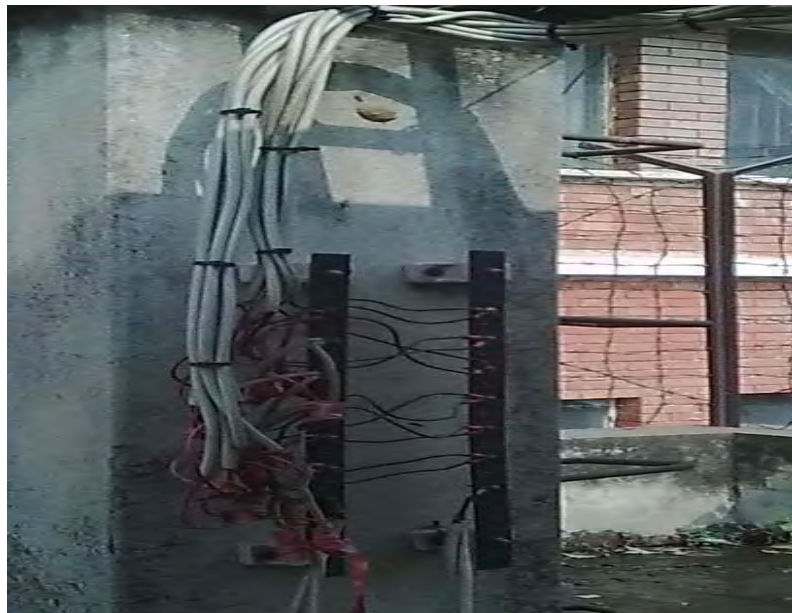
Figure 4.2: Combiner Box connection from Solar Array
