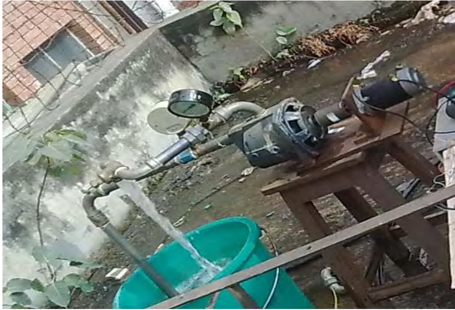
Figure 4.3: DC motor and Pump Set
