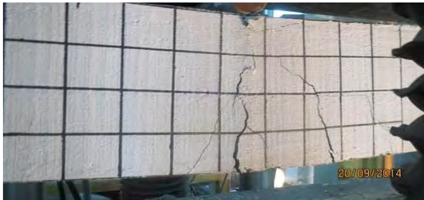
Figure 4.27 Failure Pattern of Specimen-HB53PC
