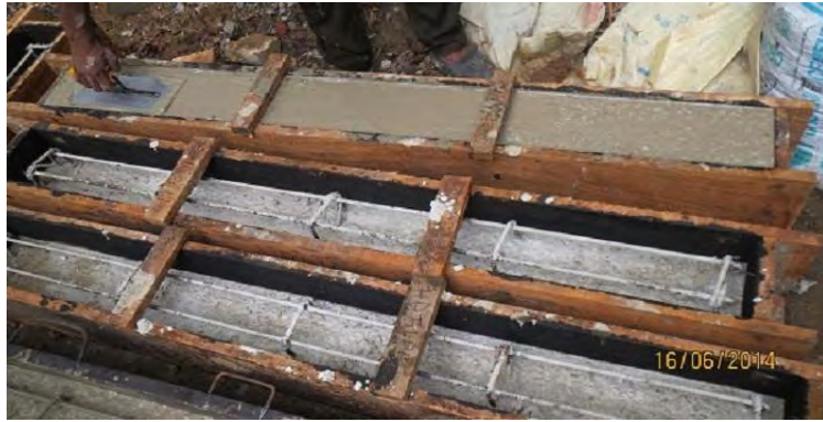
Figure: 3.11 Half Made Beam Was Fully Cast Without Using Any Bonding Agent After One Day
