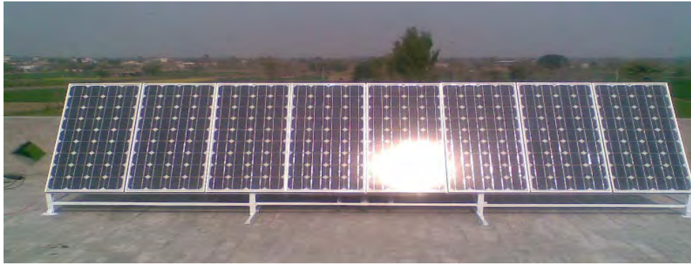
Figure 3.15: Solar array (series of modules)
