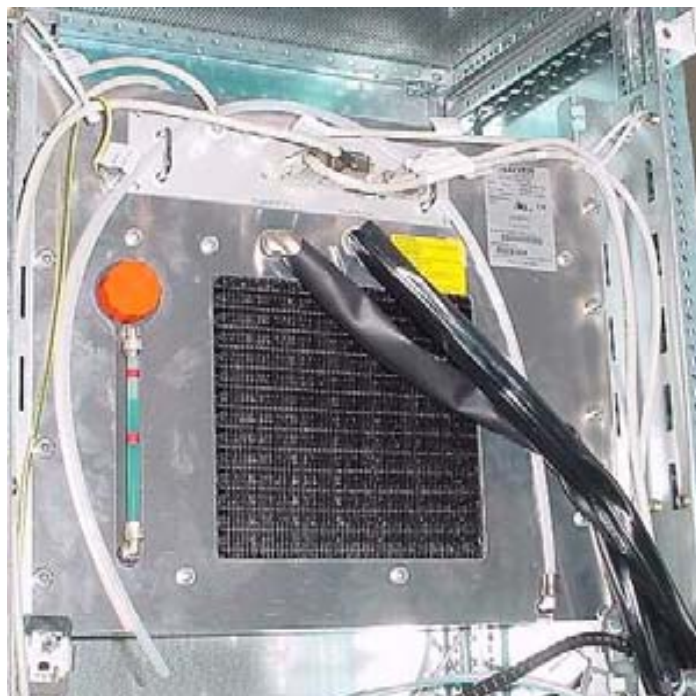
Fig 4.11: Detector cooling Unit
