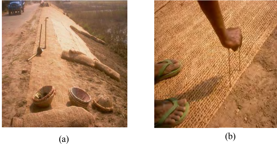
Figure 4.29 Geo-jute laying; (a) roll placing at site, (b) attaching geo-jute with U hook
