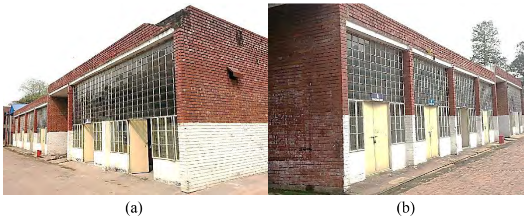
Figure 4.5: Views from (a) right side and (b) left side of the Building No. 6C
