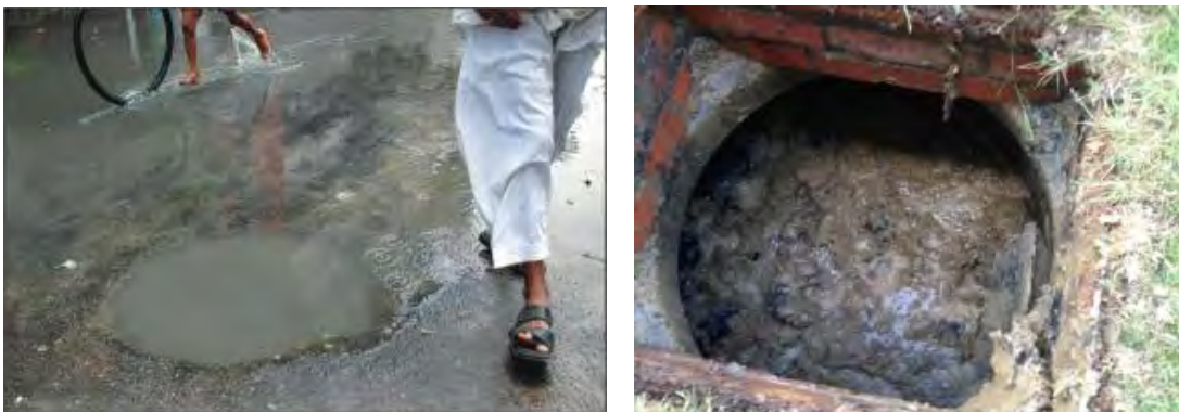
Fig. 4.10: Blockage in Manholes and Catch Pits
