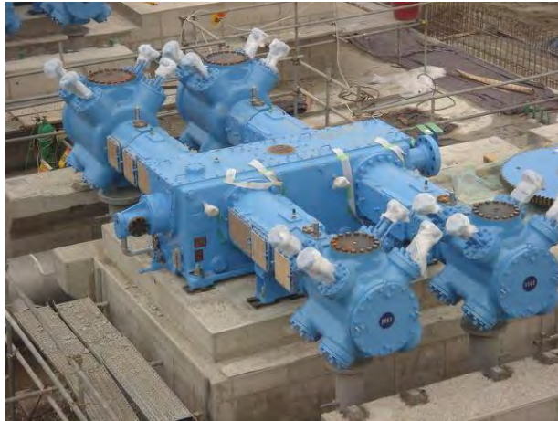
Figure 3.5: LNG Boil off gas (BOG) compressor (Source- blog.daum.net)
