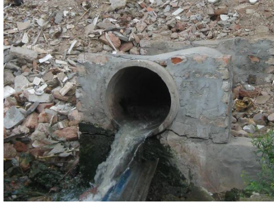
Fig 3.7: Stains inside pipe, near Moriom Tower-1
