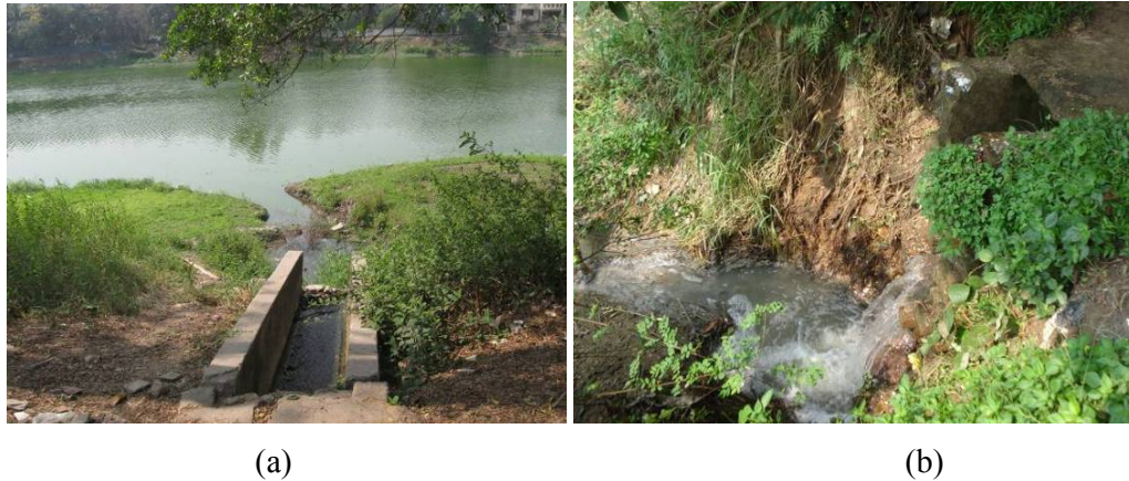
Fig 3.2: Open outfalls in first segment, (a) drain near R#6 and (b) drain near R#4
