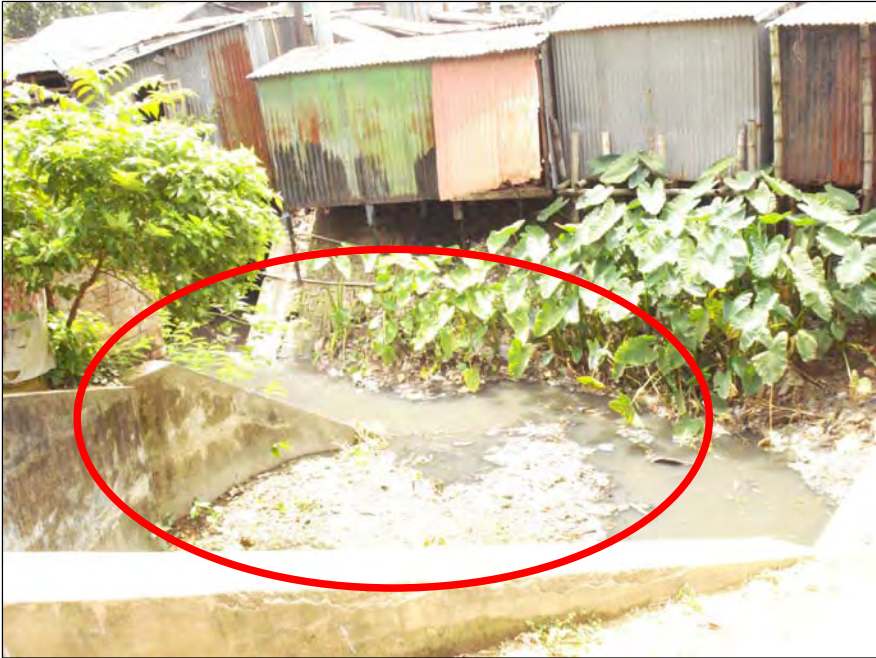
Plate 7.14: Garbage carried by drain deposited at entrance gate of sluice gate
