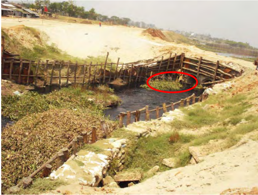
Plate 7.10: Garbage deposited at the entrance of Pipe culvert in the under construction road
