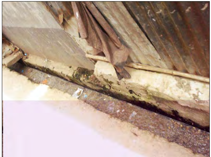
Plate 7.2: Drains are rarely cleaned
