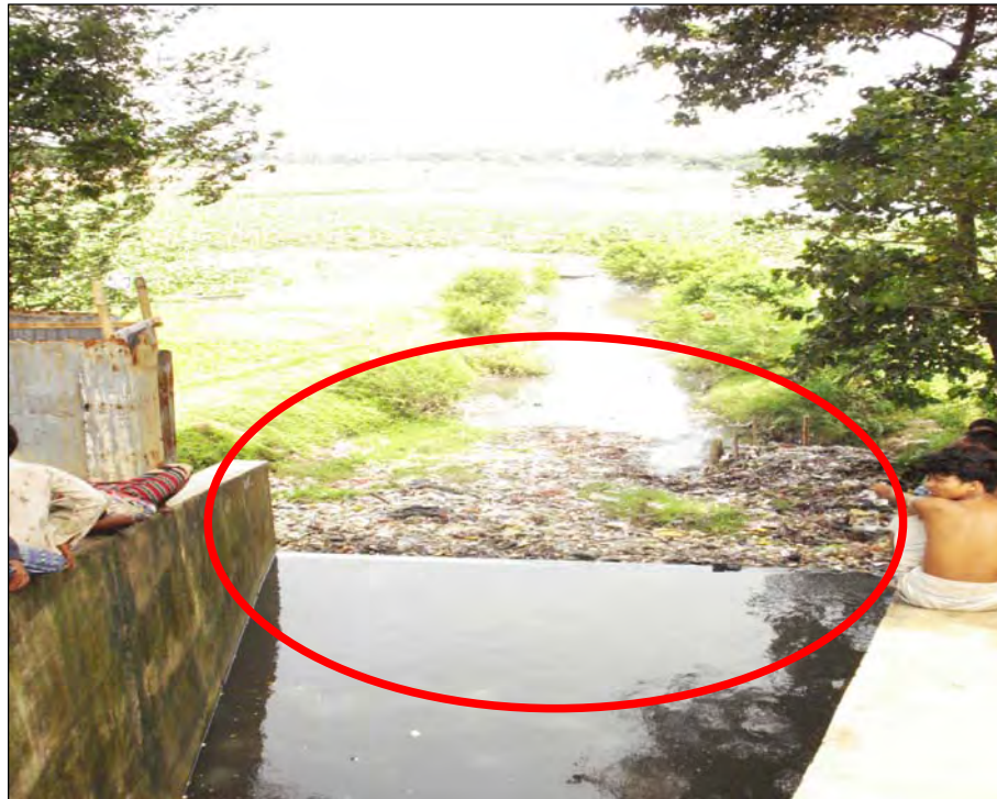
Plate 7.15: Garbage carried by drain deposited at exit gate of sluice gate
