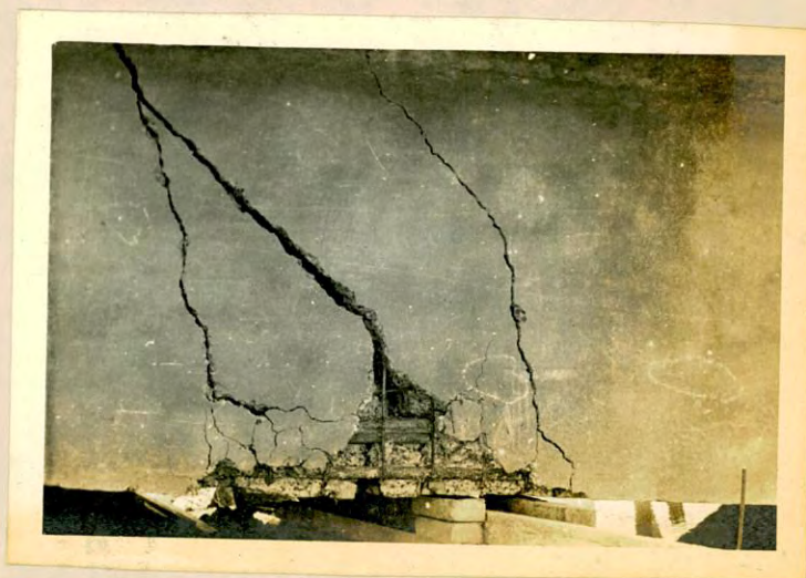
Plate 2.5 Mathabhanga Bridge (Cracks in the girder due to impact on falling)
