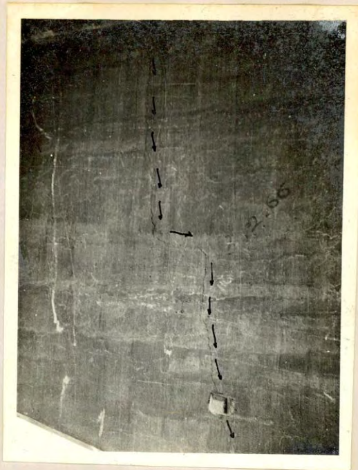
Plate 5.2 C Tongi Bridge (Crack in the upstream main girder; the wide crack is vertical, then horizontal and vertical again at the bottom)
