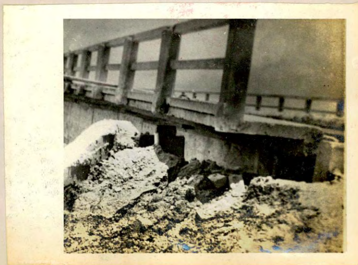
Plate 6.1. B Failure of the wing-wall
