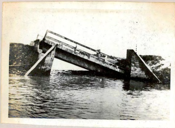
Plate 6.3 Failure of abutment (Abutment collapsed, but wing-wall remained in position)
