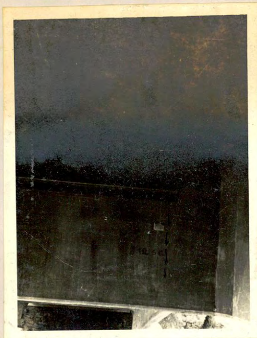
Plate 5.2 B Tongi Bridge (Crack in the cross-girder at articulation, showing the bolts that connected two opposite cross-girders at articulation)
