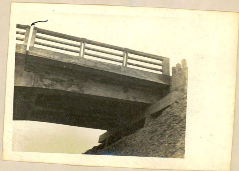
Plate 6.10 Failure of abutment reflected at articulation
