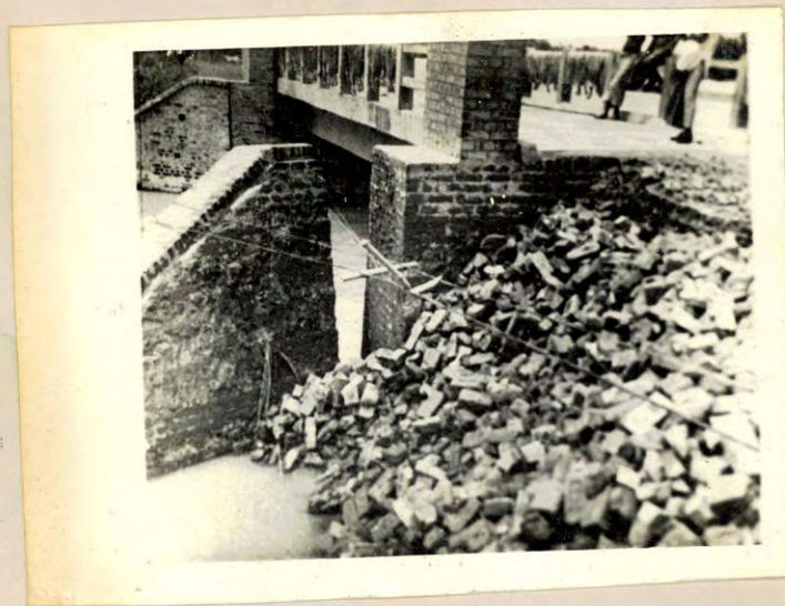
Plate 6.4 Failure of wing wall
