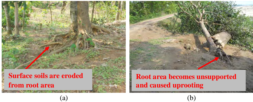
Fig. 2.3 (a) Erosion of surface layer uncovered root area and (b) uprooted tree
