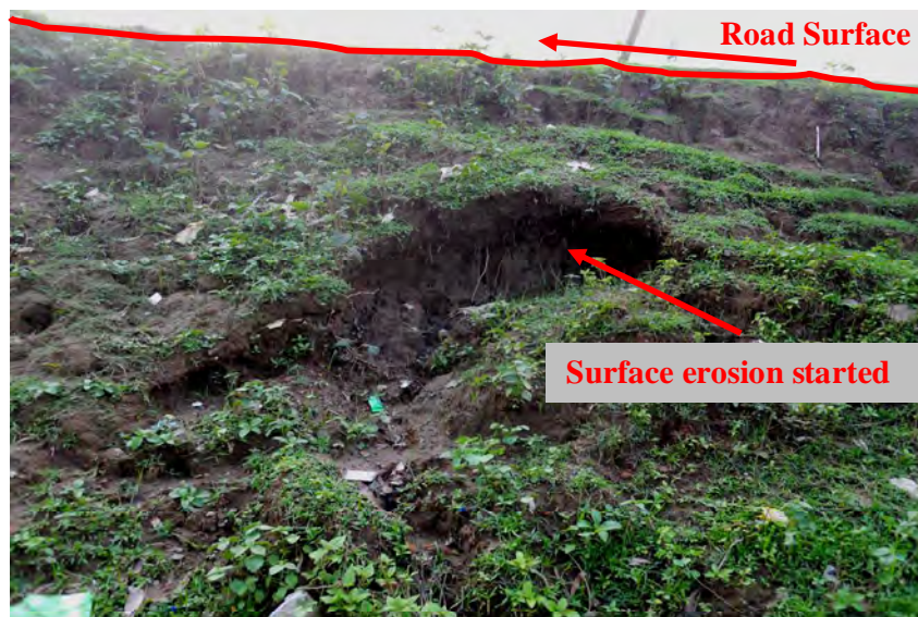
Fig. 2.1 Surface erosion in road embankment
