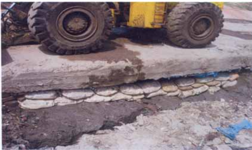
Figure 2.10: Prevention of collapse of Road (BRTC, 2008)
