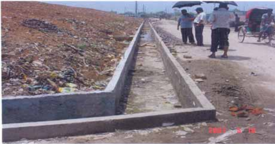
Figure 2.12: Storm Water Drainage System In front of the Control Area (BRTC, 2008)
