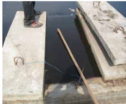
Submerged condition of leachate pond
