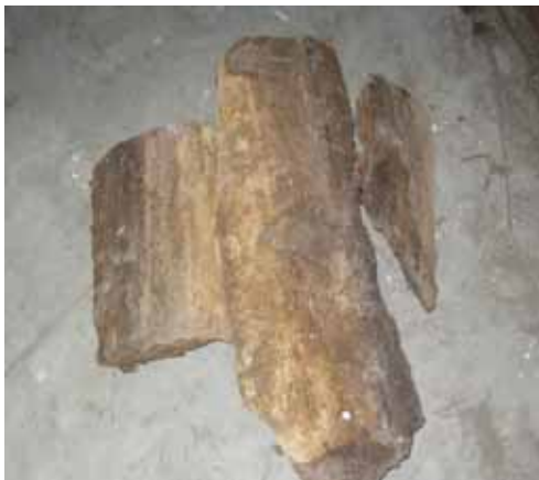
Deposited iron shell in leachate pipe
