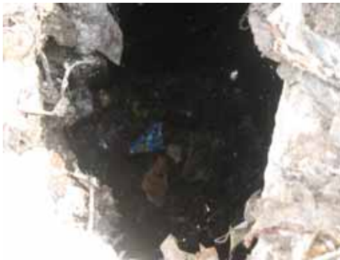
Poor maintenance of drainage pit
