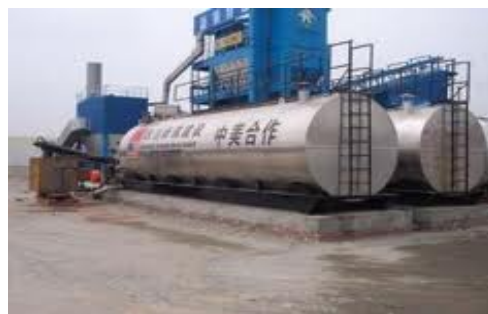
Figure 3.1: A VSS asphalt rubber blending system in China.
