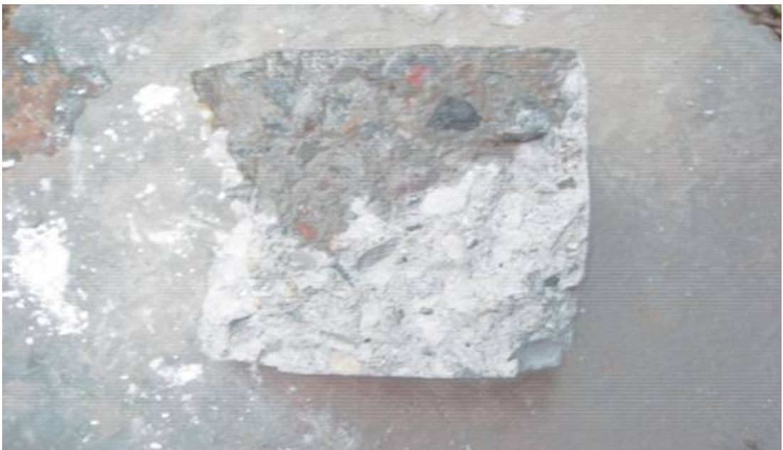
Fig-A9: Wet surface (stone aggregate concrete)
