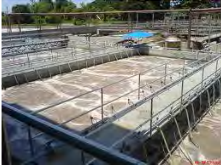
Figure 2.3. Aeration tank in operation
