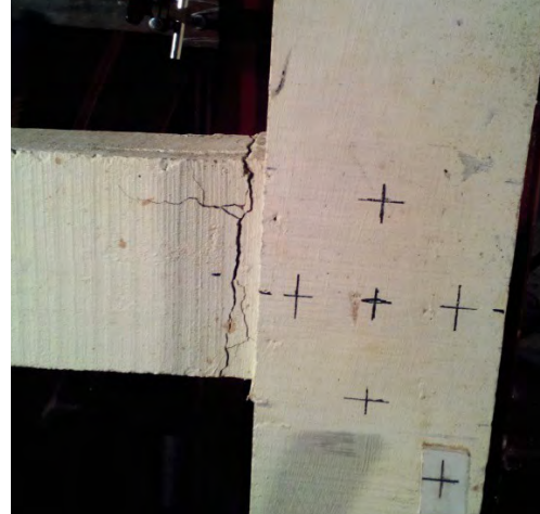
Fig. 5.6: Appearance of Shear Crack
