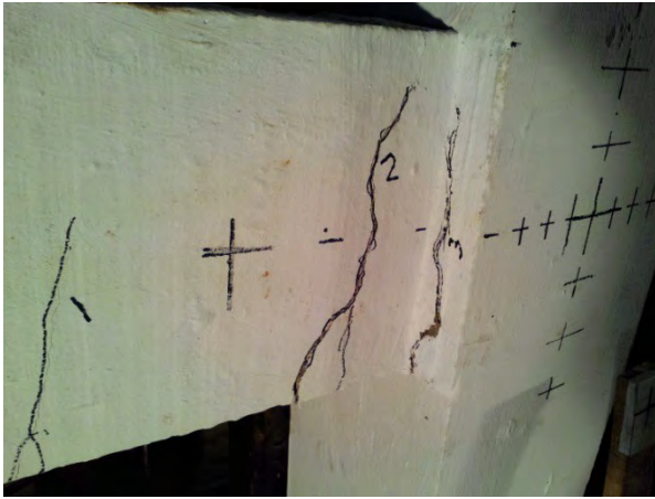
Fig. 5.3 : Shear Crack at Column Joint Face
