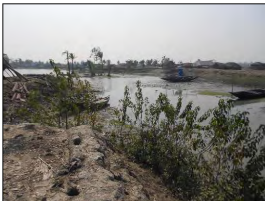
Photo B1: Damages to embankment by Aila.
