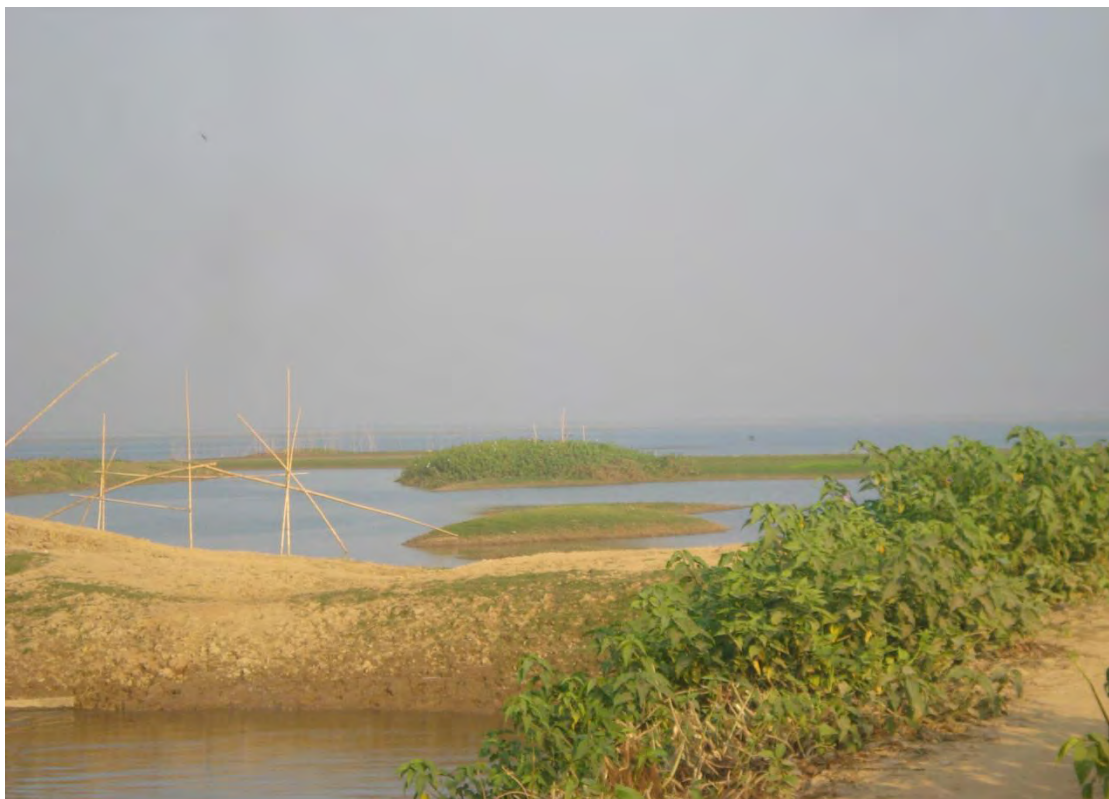
Photo 5.3 Condition of submersible embankment at Zirak Tahirpur after flood
