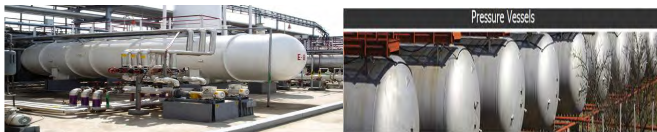
Fig-3.3 Pressure vessel [21];
