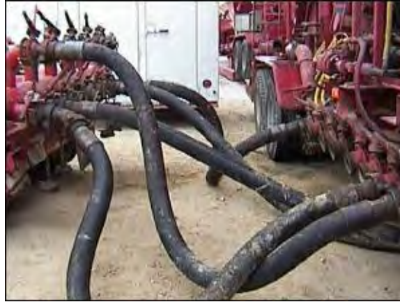
Fig-3.16 High Pressure Lines and Equipment, [10];
