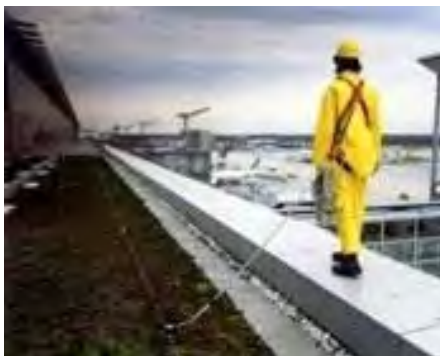
Fig- 4.31 The worker is protected by a properly constructed fall arrest system [52];
