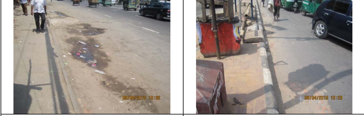
Bad drainage facilities at intersection
