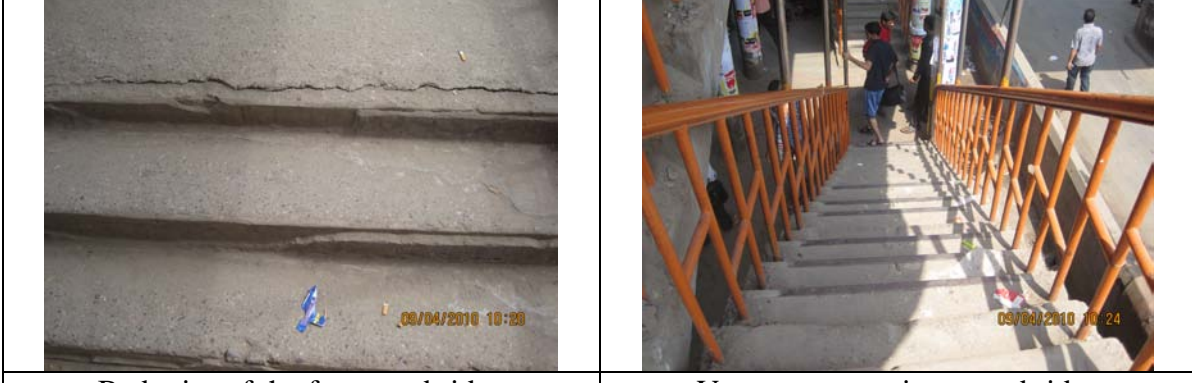
Bad raise of the footover bridge
