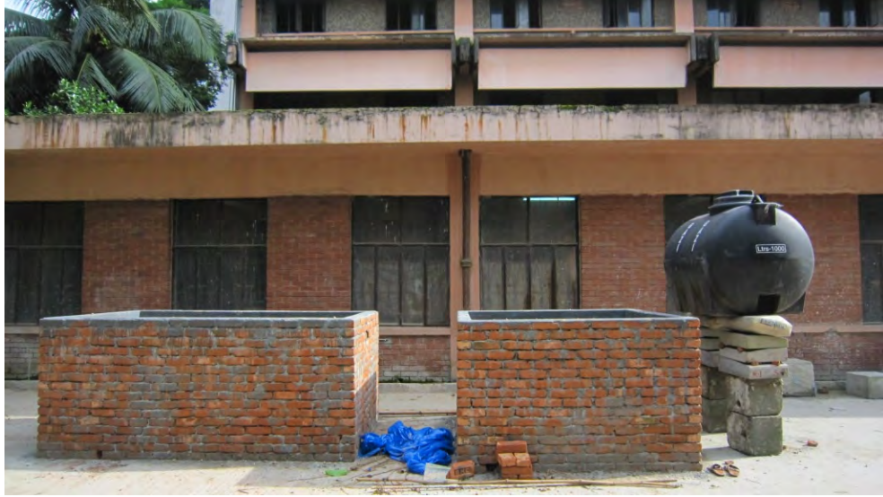
Figure 10: Two subsurface flow constructed wetland basins at BUET.
