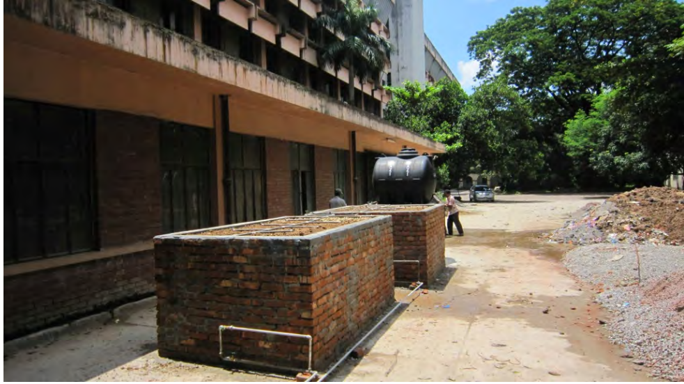
Figure 12: Constructed wetlands with pipe networks from the grey water reservoir to collection tank.
