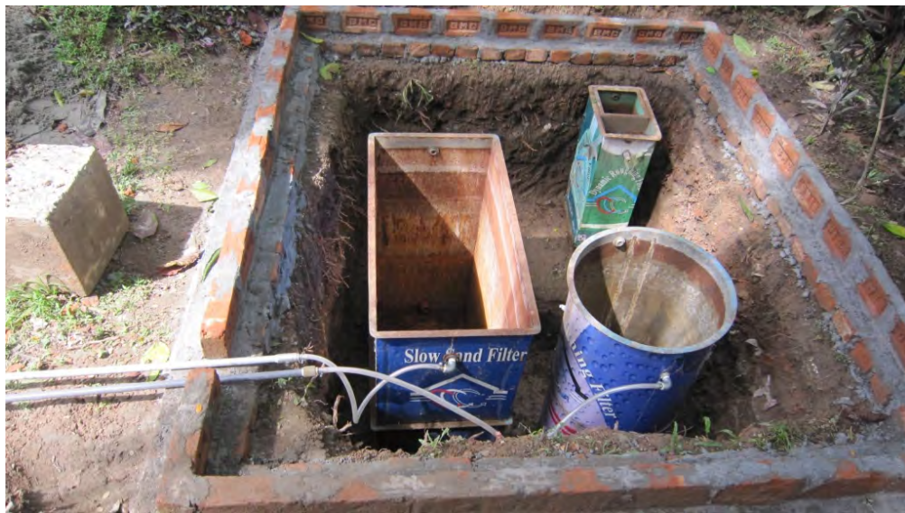
Figure 11: Collection system to collect treated grey water from wetland basins.
