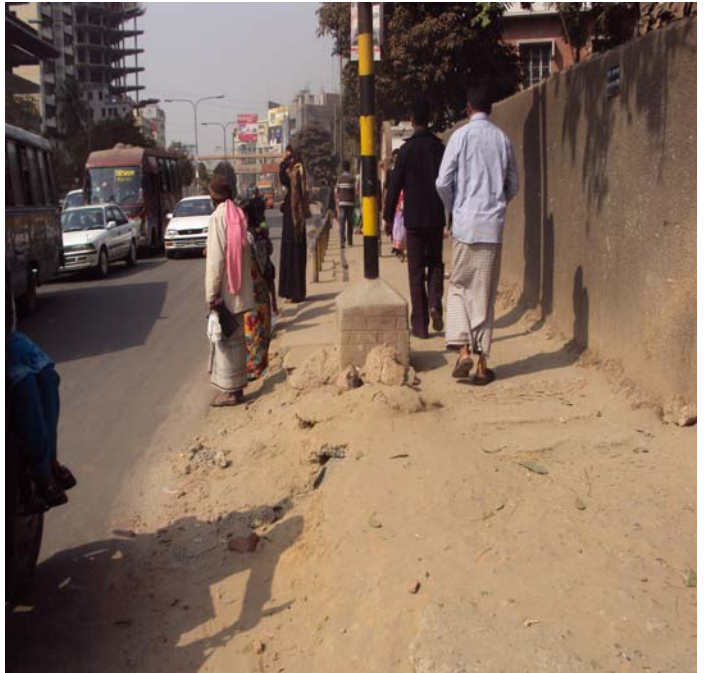
Figure 18: Broken Footpath in ShishuMela Intersection
