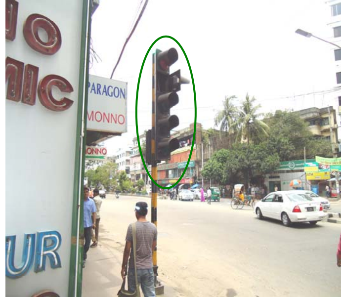
Figure 2: Signal Head Broken in Bata crossing intersection.
