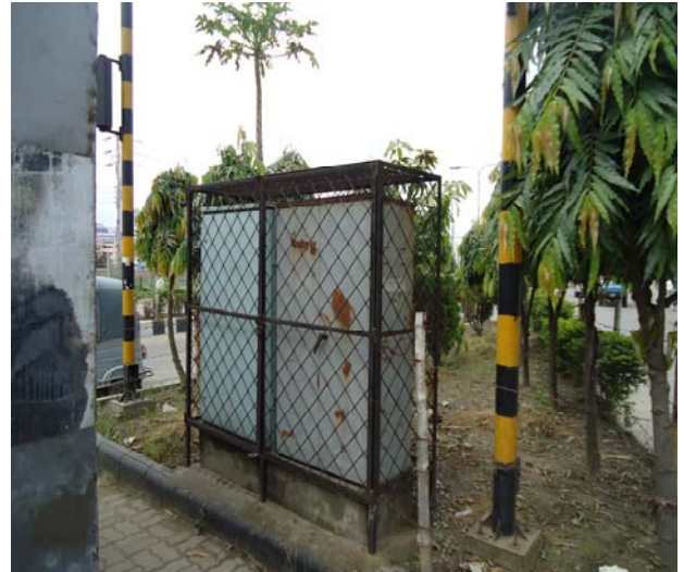
Figure 4.5 d: One Controller Cabinet is Corroded in Tongi Diversion Intersection.
