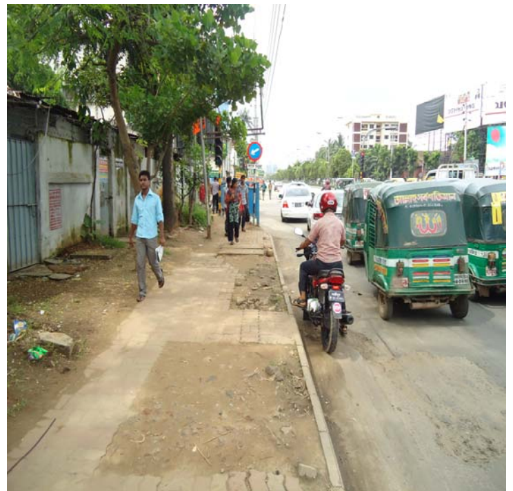
Figure 8: Broken Footpath in Tejgaon Rangs Link Road Intersection.
