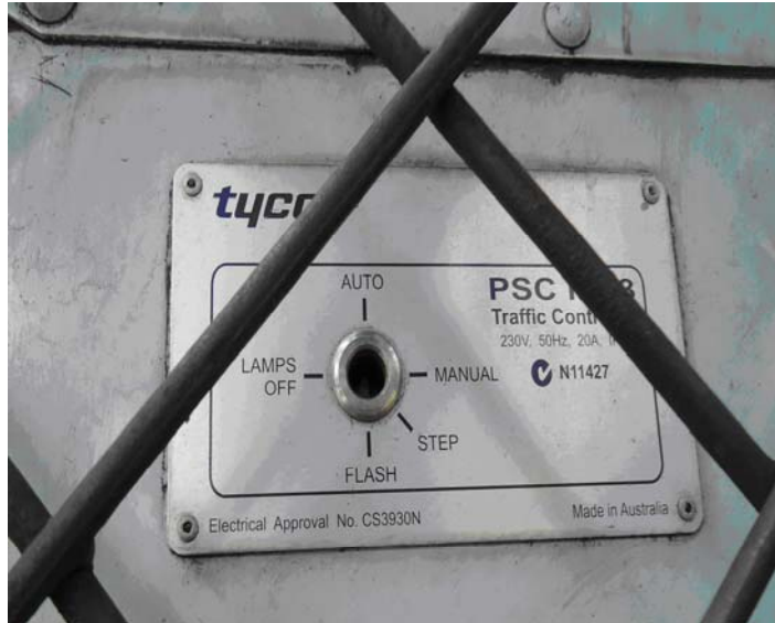
Figure 4.44: Manual Control Key in Controller Cabinet at Jahangir Gate.
