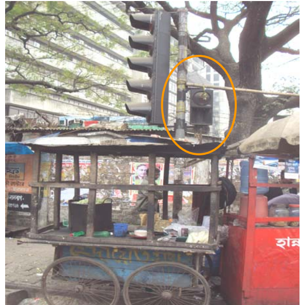
Figure 4.25b) Pedestrian signal head Broken at Dhakashori approach in Palashi
