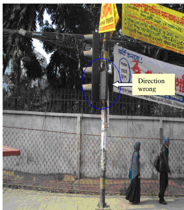
Figure 4.24 b) Pedestrian signal head condition in Bashundhara Intersection
