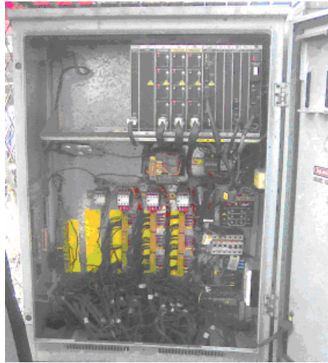
Figure 4.45: Typical Controller Cabinet
