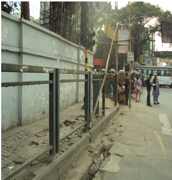
Figure 4.28a) Footpath Condition at East Approach in Azimpur Intersection.
