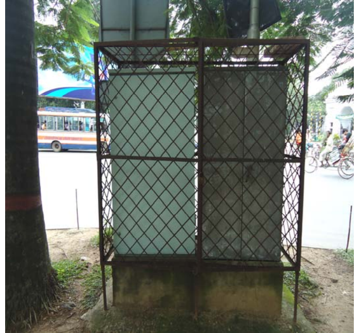
Figure 6: One Controller Cabinet is Colorless in Curzon Hall Intersection.
