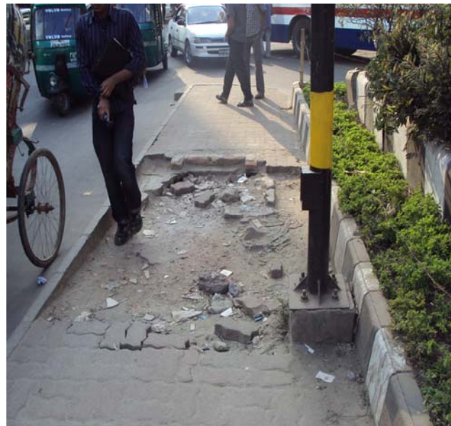
Figure 4.28b) Broken Footpath in Gulshan- 1 Intersection
