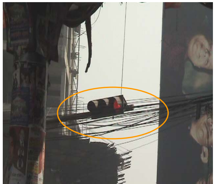
Figure 4.32f): Cable in front of primary signal at Mouchak
