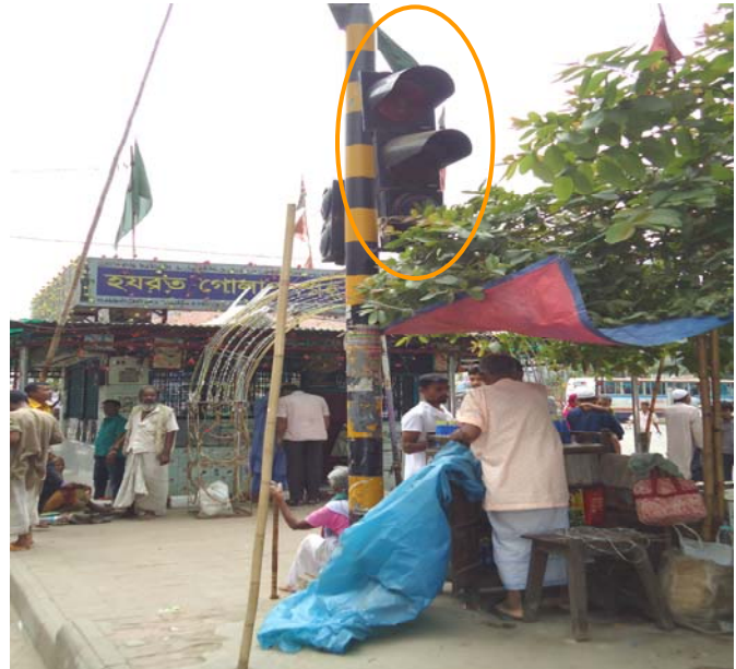
Figure 4: Signal Head Broken and not vertical in Gulistan/Golapshah Mazar
