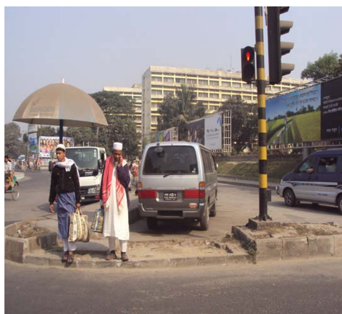
Figure 4.30b) Pedestrian refuge broken at Khamarbari
