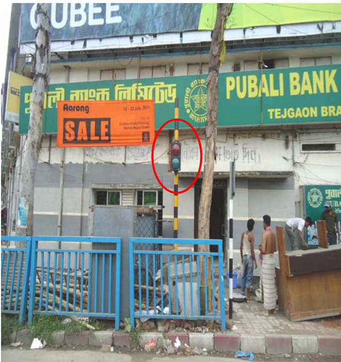
Figure 7: Pedestrian Signal Light is Off in Tejgaon Rangs Link Road Intersection.
