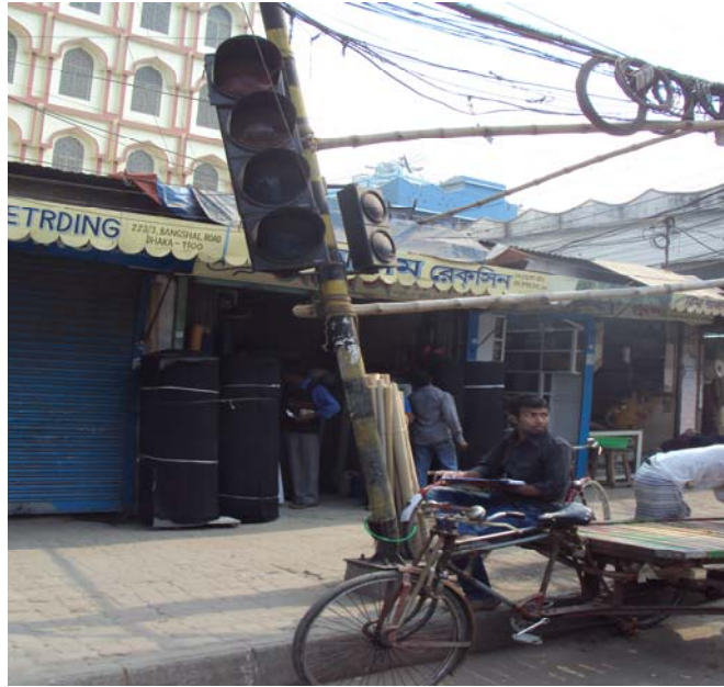
Figure 4.9: Signal Pole Condition in Bangshal Intersection.
